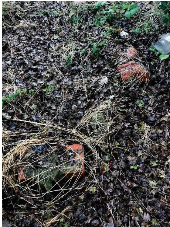
Photo 8: Building waste in southwest corner of site
