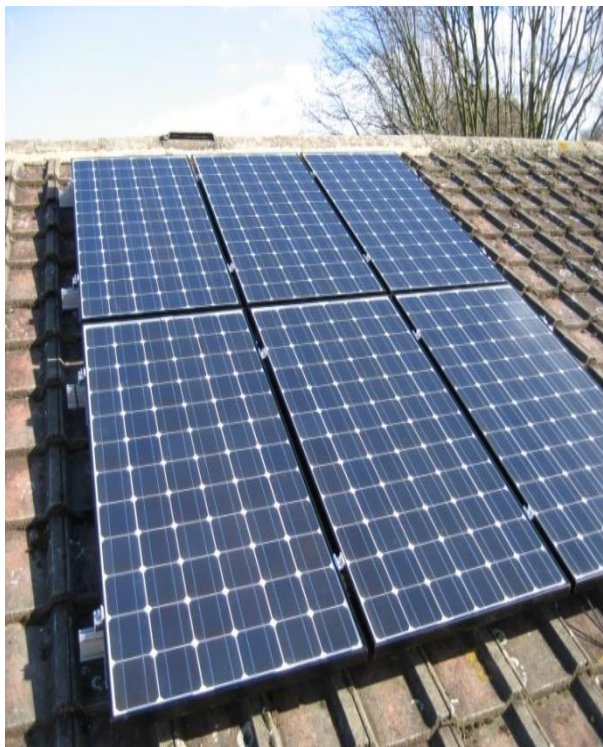
Figure 6 - Photovoltaic array on a pitched roof
