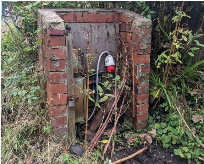
Figure 3 – An industrial electric outlet for buildings along the western site boundary, looking south-east.
