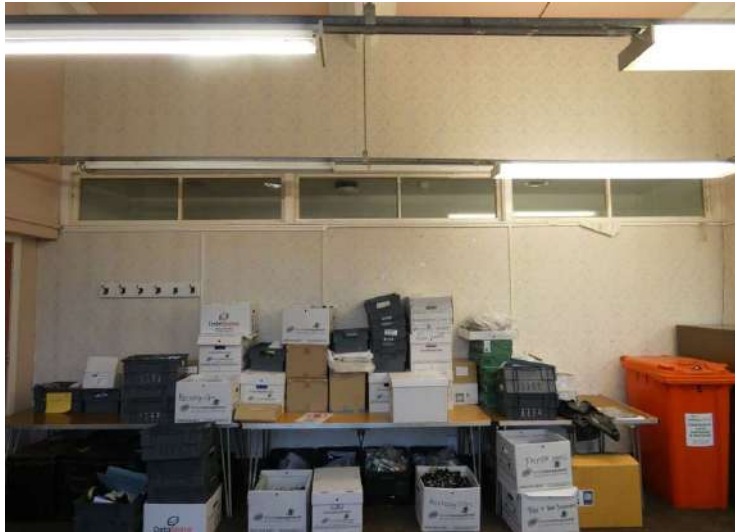
F6c. View west, the inserted partition cuts accross historic features.
