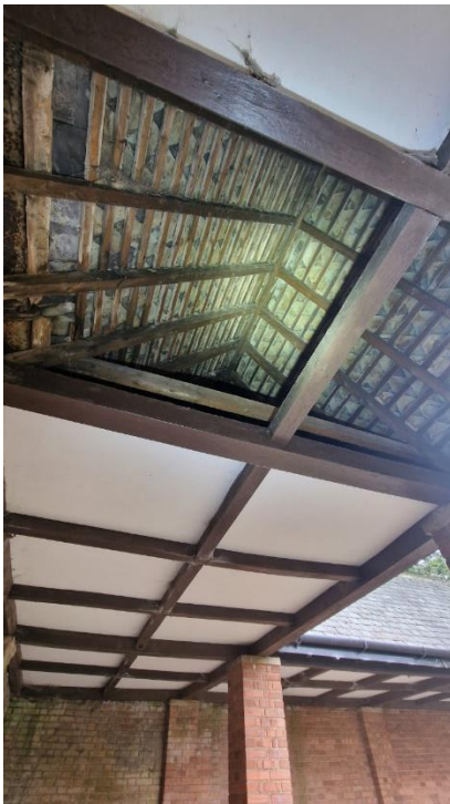
6. Missing ceiling panels
