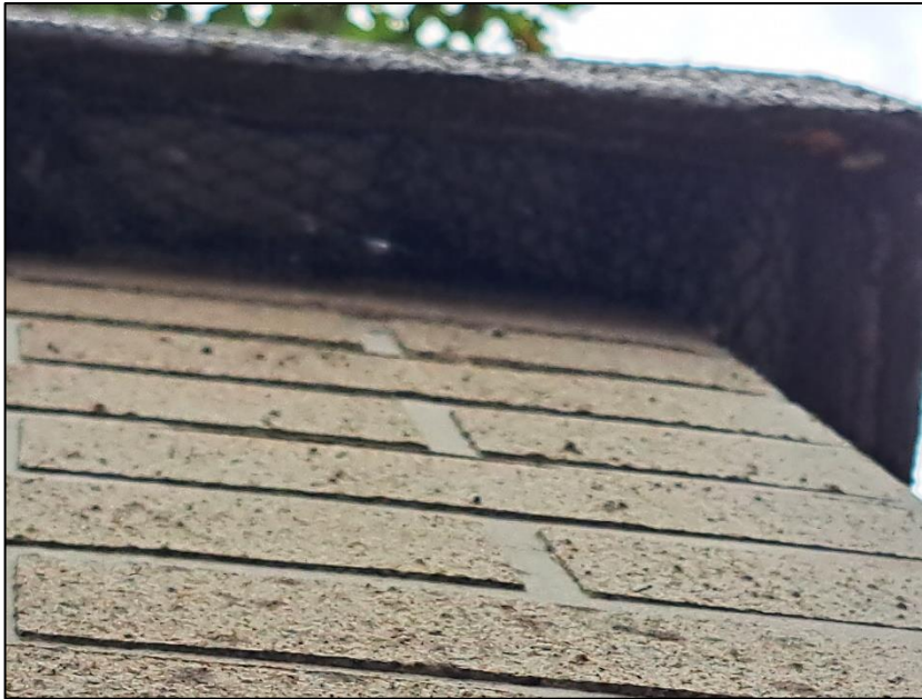
Photograph 18 showing the large gap between the top of the wall and the roof overhang
