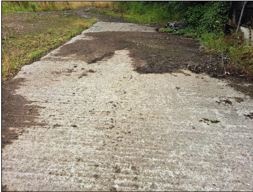
Photograph 6 showing an area of bare ground at the site entrance
