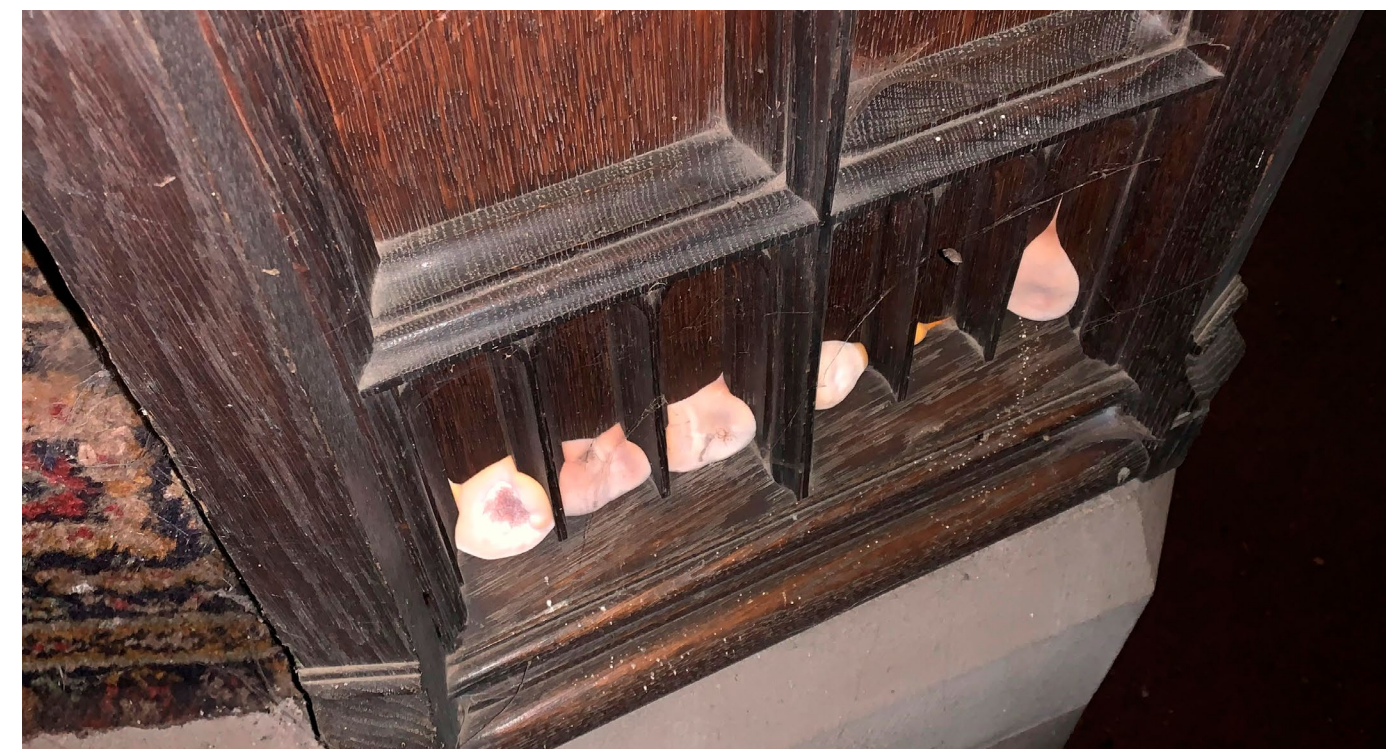
Figure 27 Images of Dry Rot Fungus on Pulpit
