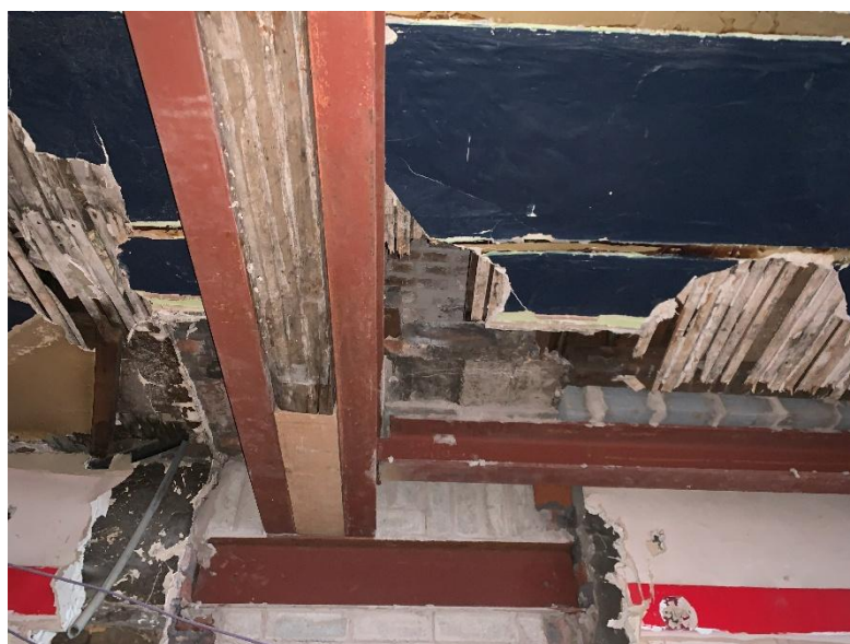
Figure 2.5: Timber beam reinforced by steel, and damaged lath and plaster ceilings.
