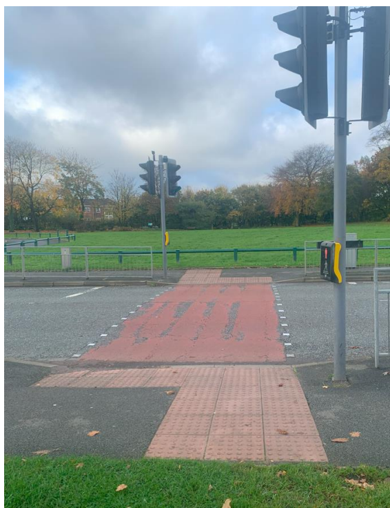
Photograph 9: Norden Road Signalised Crossing
