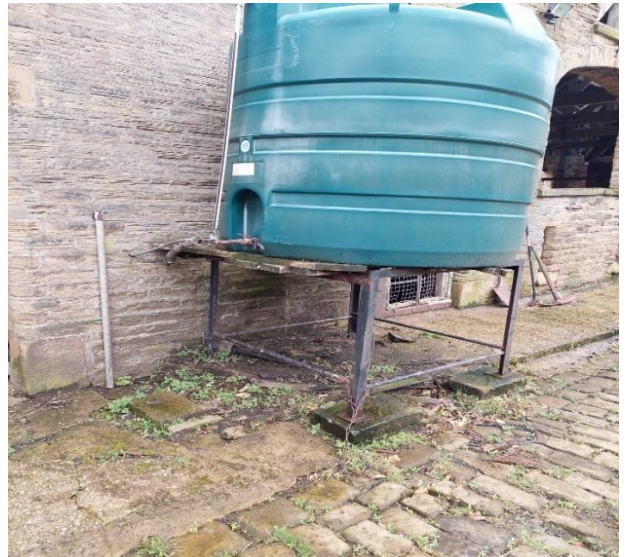
Photograph 6: Oil heating tank in cobbled courtyard
