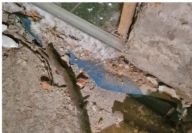
Blue DPM showing under the storage room screed.
