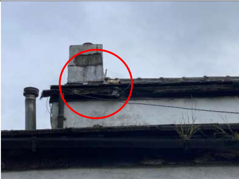
Figure 9: Damaged mortar on the chimney stack visible from the northern elevation of B1. Also visible are lifted lead flashing at the base of the chimney stack.
