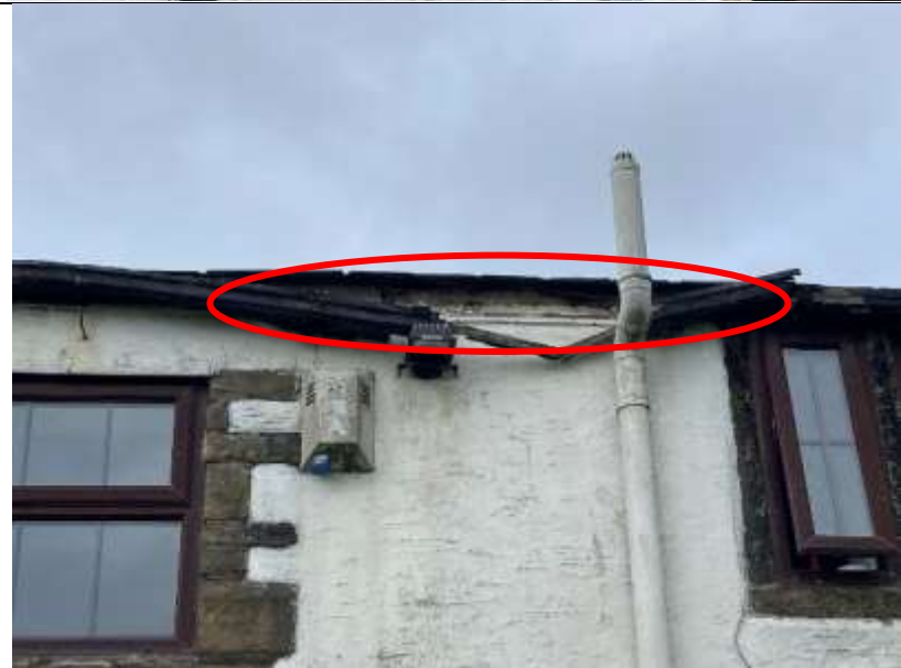
Figure 8: Damaged fascia boards on the southern elevation.
