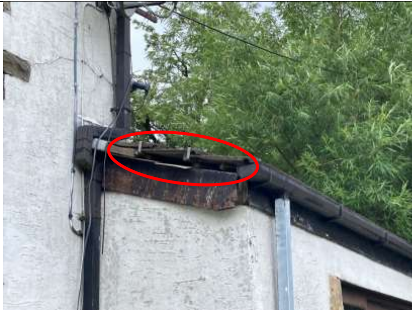
Figure 7: Missing mortar under field tiles on the porch extension located on the southern elevation of B1.
