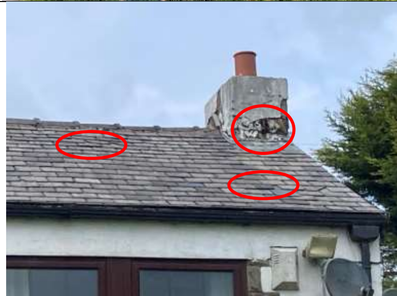
Figure 6: Showing the lifted field tiles and missing/damaged mortar to the chimney stack of B1.
