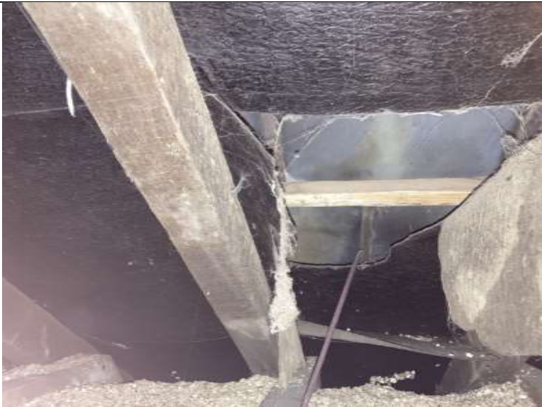
Figure 15: Showing the damage to bitumen felt lining within internal void 2.
