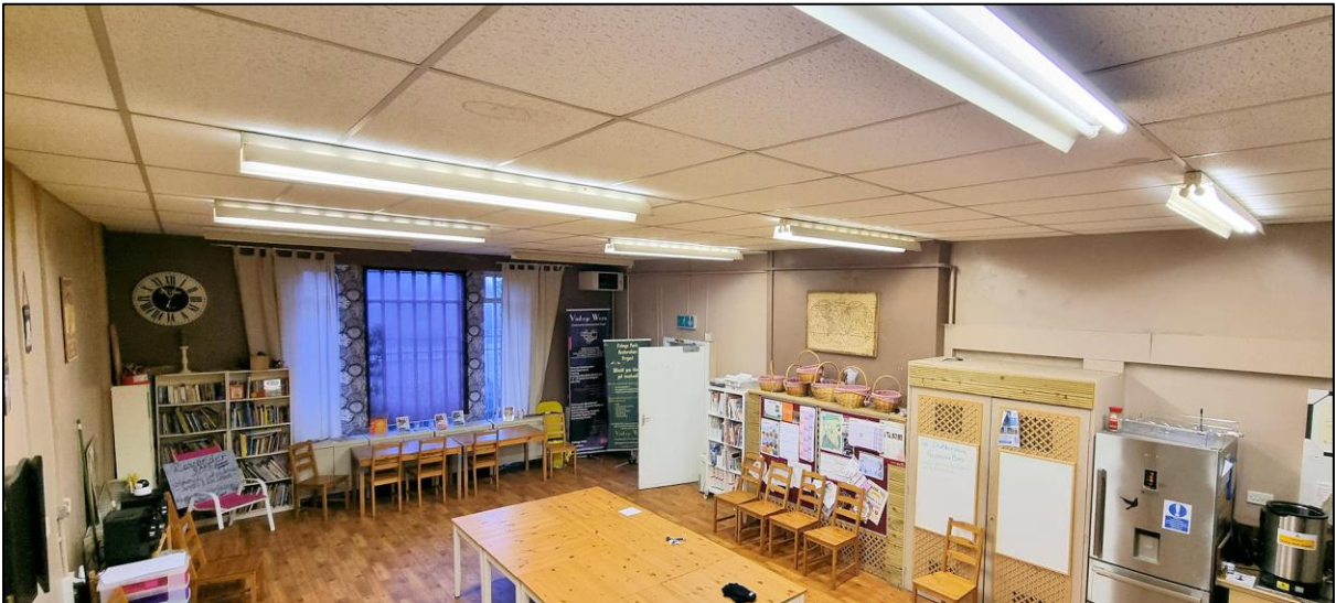
Plate 23: The suspended ceiling of the east pavilion was intact and prevented bats accessing the rooms below.
