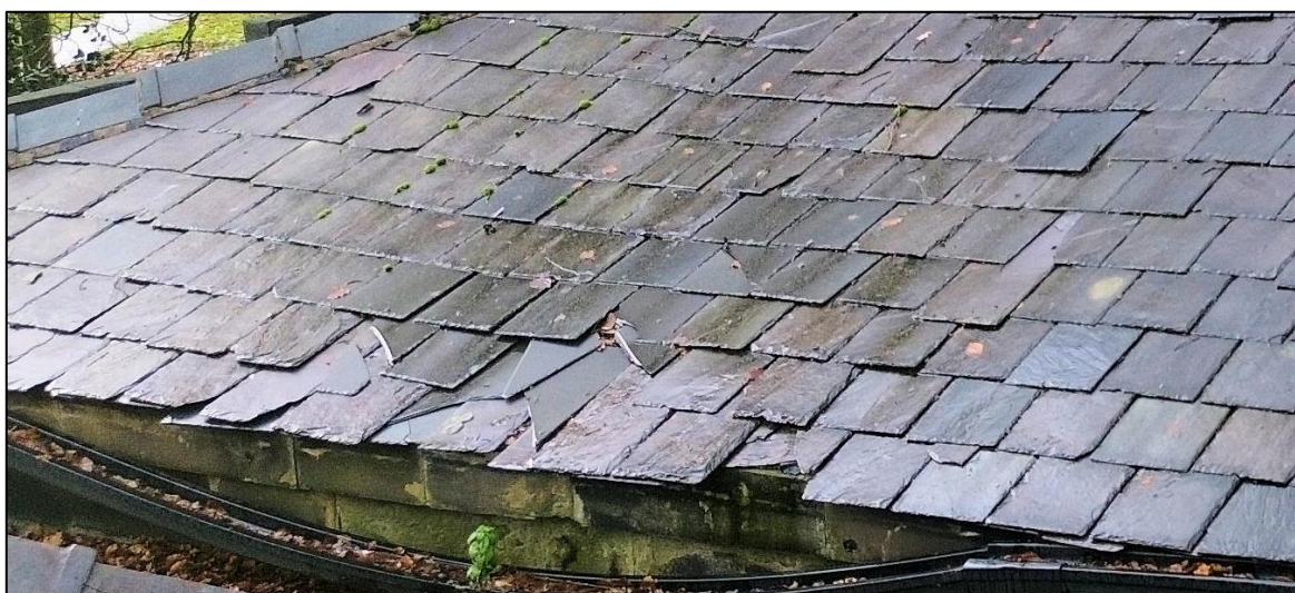
Plate 7: However, particularly on the west pavilion, there were areas of slipped and broken tiles gaps.
