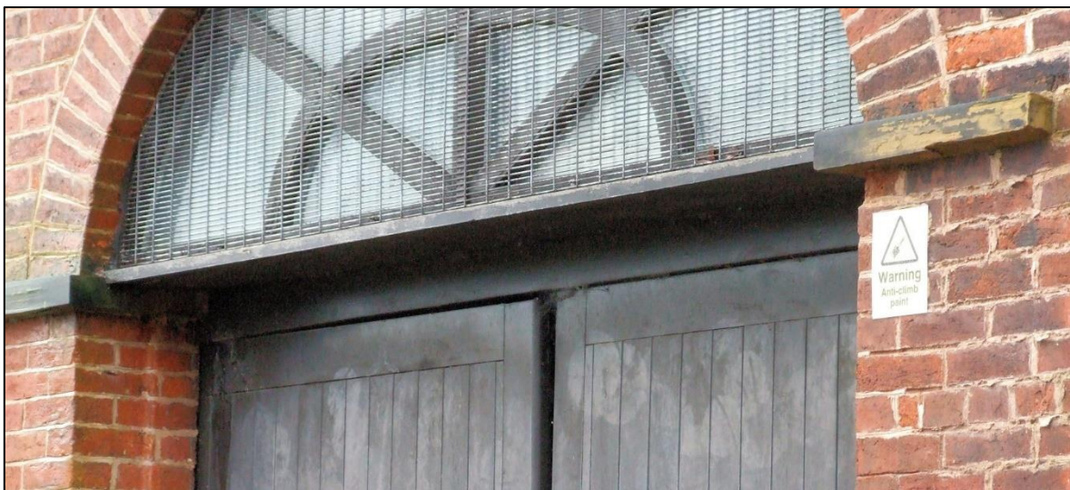
Plate 13: Although the door frames across the buildings were generally intact, there were large gaps around the doors of the Playbarn that offered potential access to the internal space.
