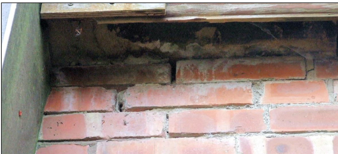
Plate 11: Although mostly intact there were gaps in the pointing of the brick walls that offered roosting potential.
