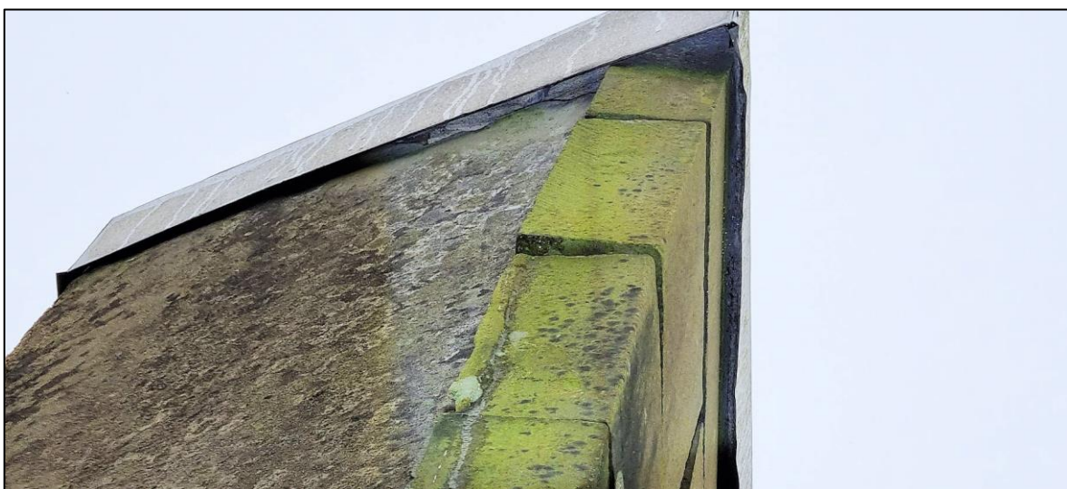
Plate 8: The roof edges were generally intact although there were gaps beneath the fascia on the newer roof of the East Pavilion.
