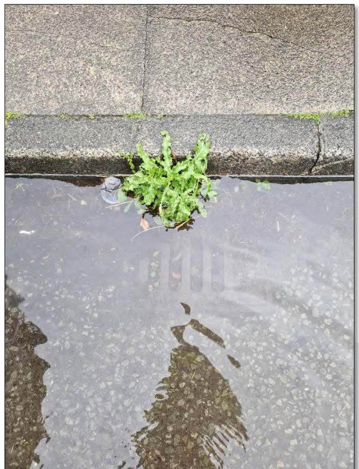
Road Gully Condition Example
