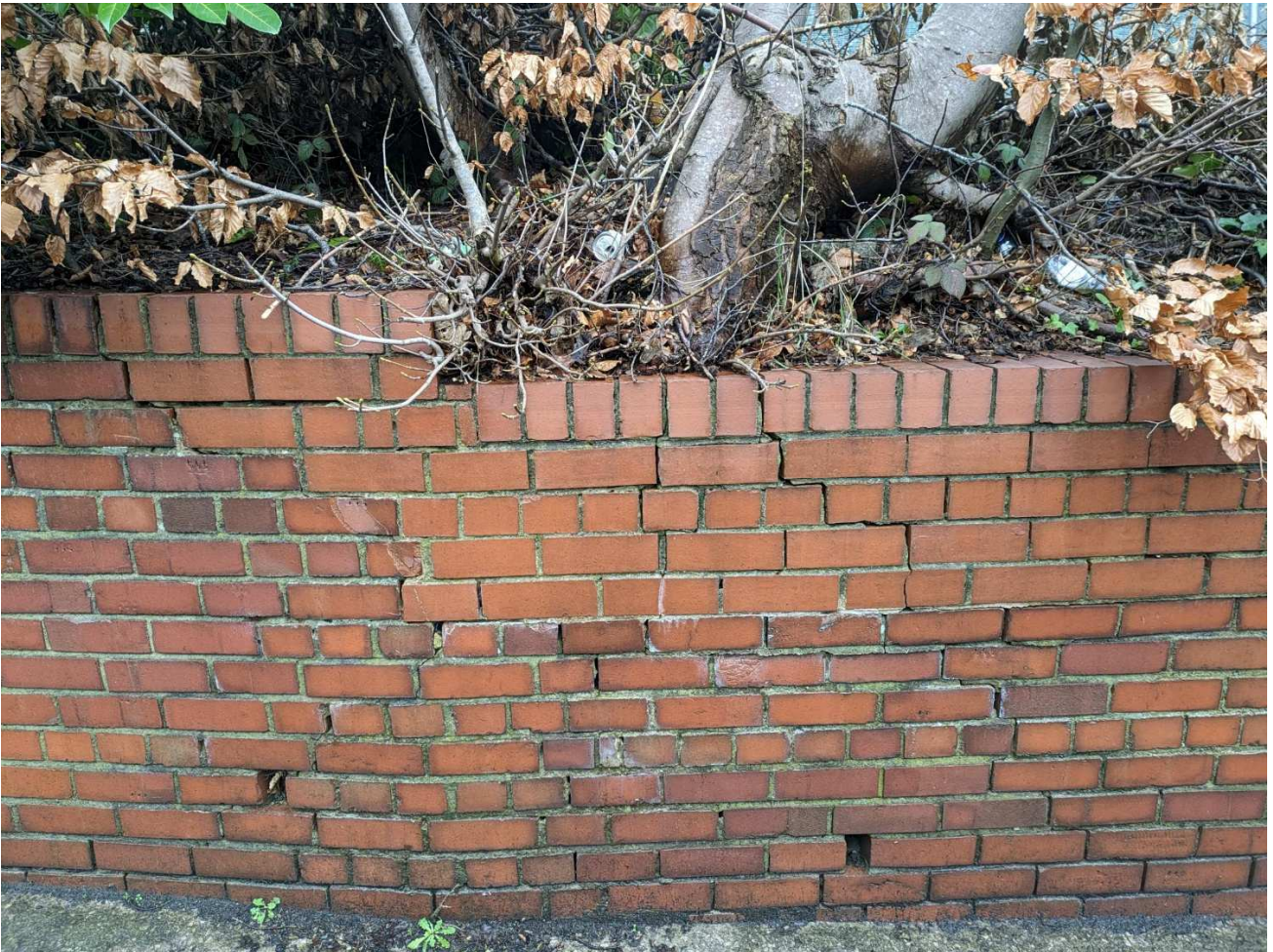
Damage to the wall adjacent to T4.
