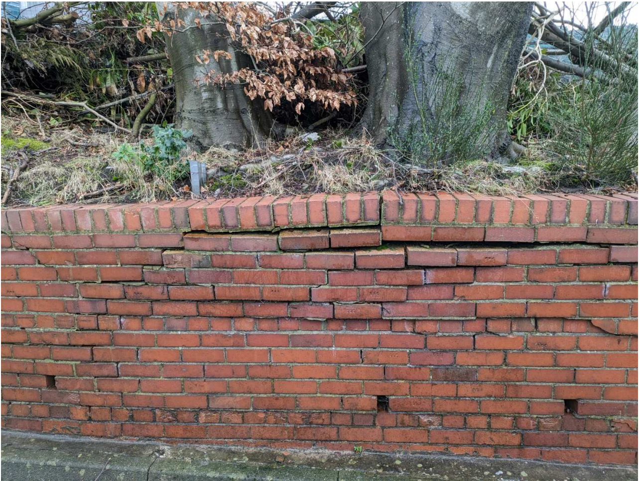
Damage to the wall adjacent to T6 and T7 .
