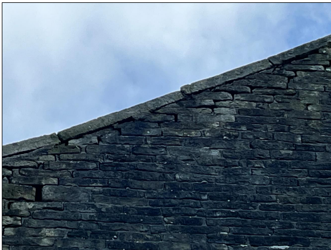
Plate 17 – Gaps in the brickwork of Section D
