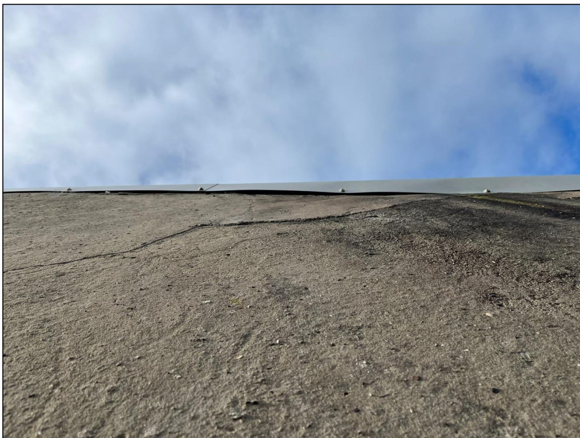
Plate 13 – Gaps beneath capping on Section A
