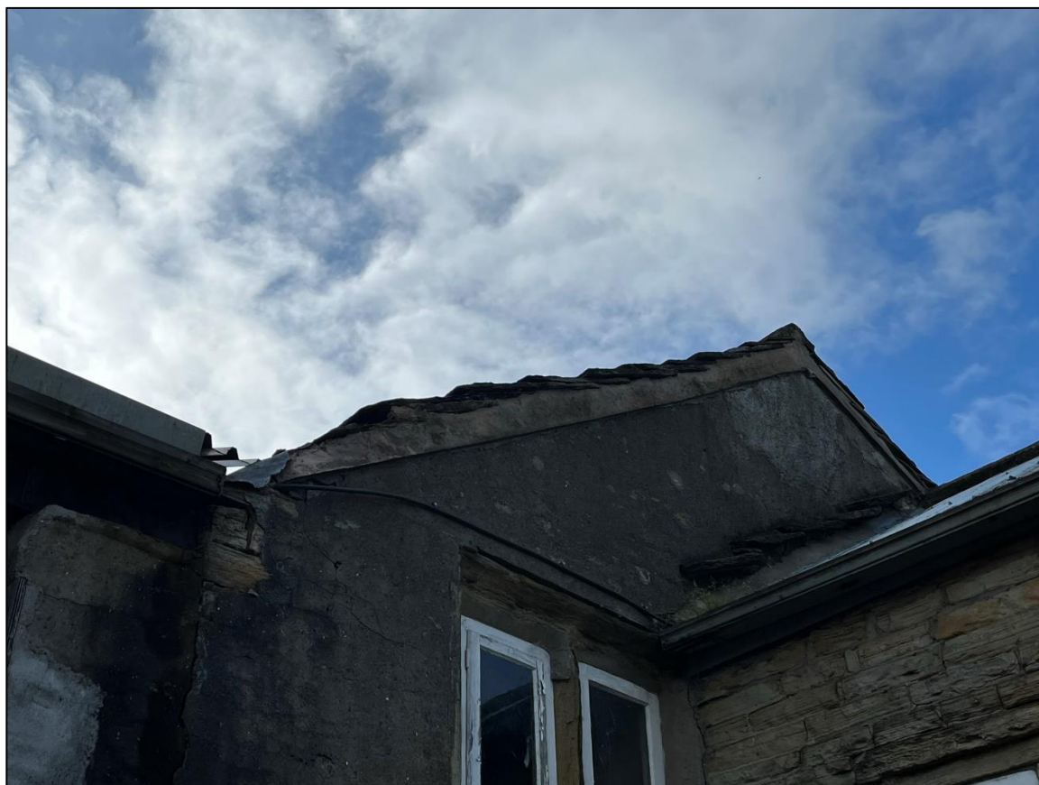
Plate 15 – Gaps beneath the slates of the gable elevation of Section B
