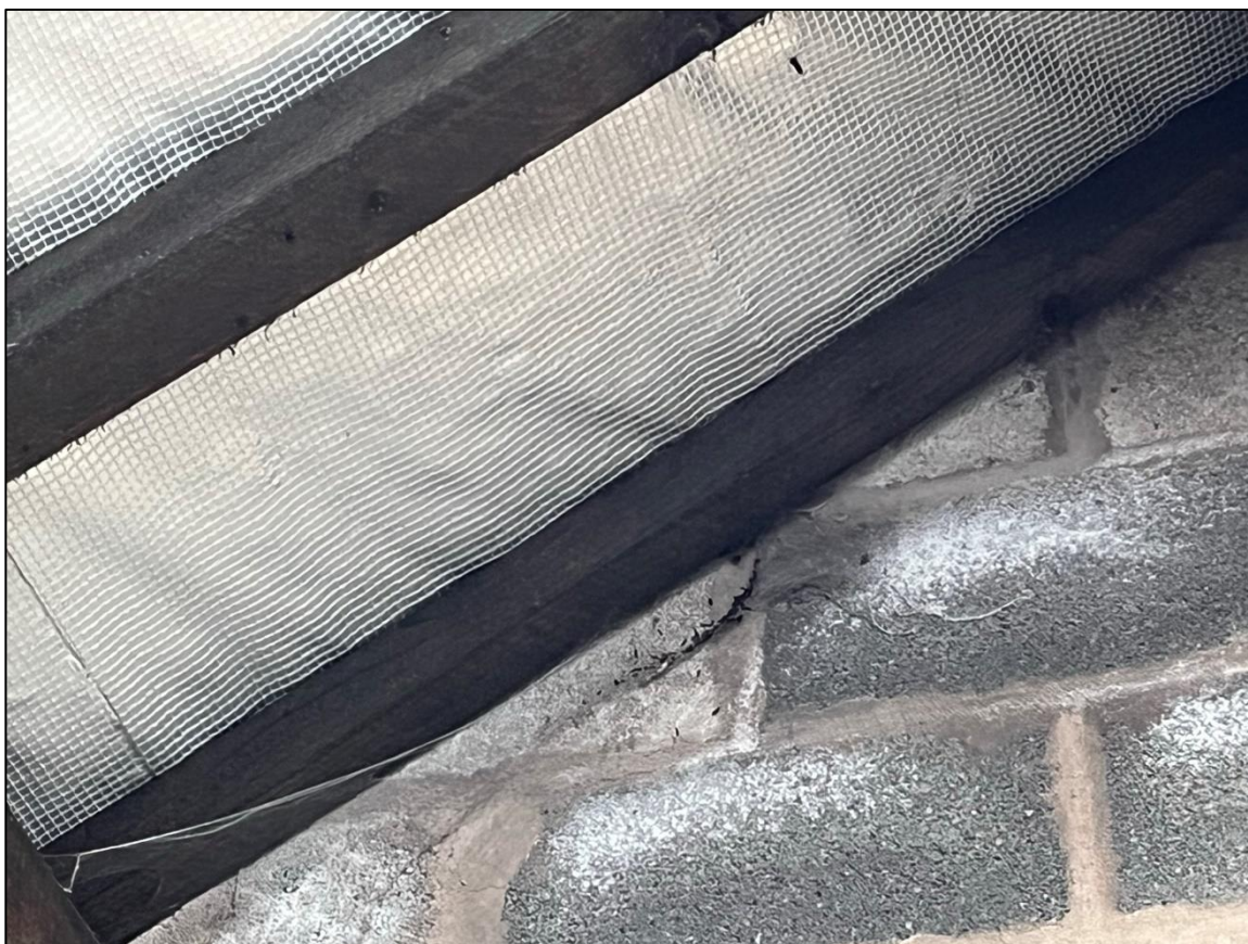
Plate 11 – Large number of bat droppings located on the gable wall of Section C
