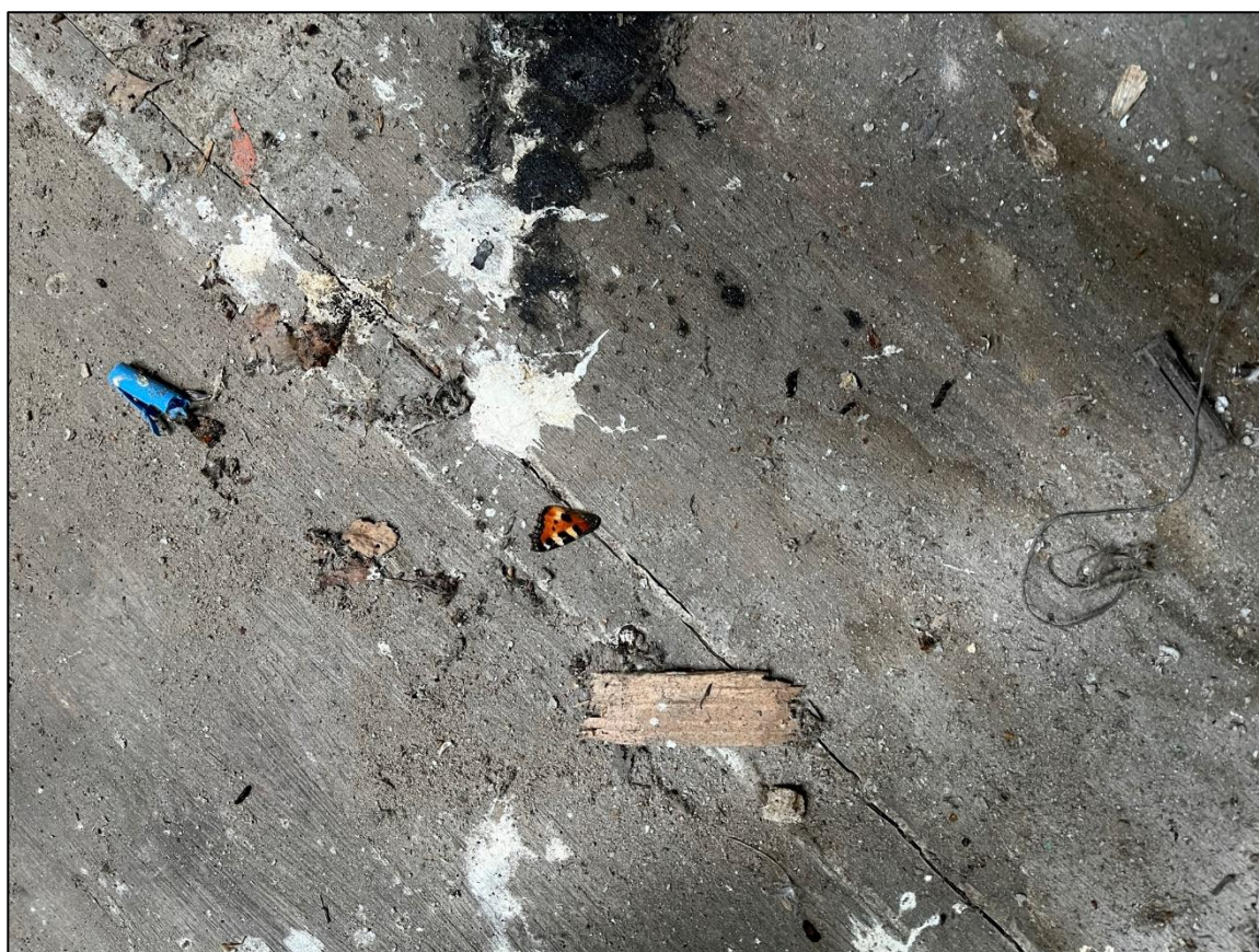
Plate 10 – Bird faecal spashing, bat droppings and feeding remains located on the floor of Section C
