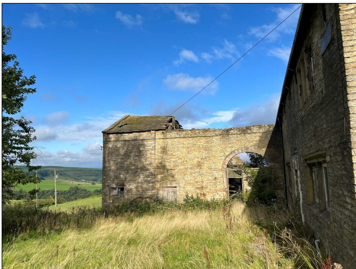
Plate 3 – Further angle of Section D, with collapsed nature evident
