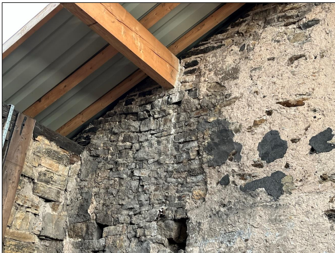
Plate 7 – Potential internal crevices within Section A
