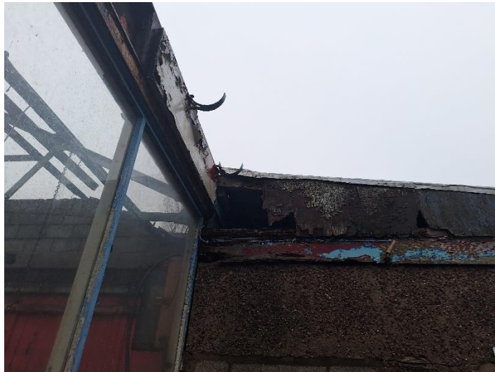
PLATE 8 SHOWING DAMAGED SOFFIT ON WESTERN ASPECT OF B1
