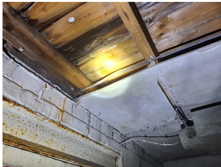
PLATE 10 SHOWING MISSING PLASTERBOARD CEILING WITHIN B1 EXTENSION
