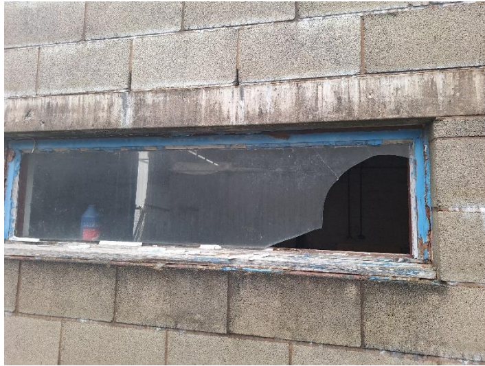
PLATE 5 SHOWING BROKEN WINDOW ON SOUTH WEST ASPECT OF B1
