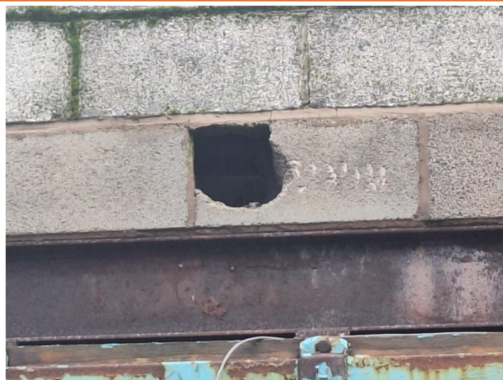
PLATE 2 SHOWING CLOSE UP OF DAMAGED BRICKWORK ON B1
