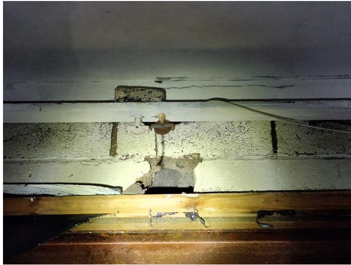
PLATE 3 SHOWING INTERNAL DAMAGED BRICKWORK OF B1
