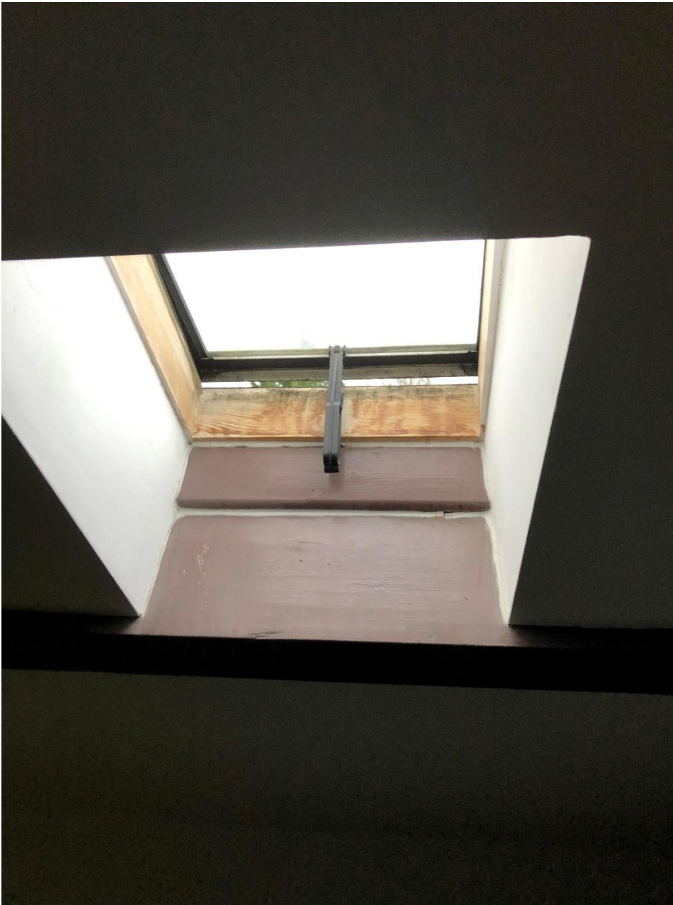
Figure 3: Picture Showing Partially Open Skylight
