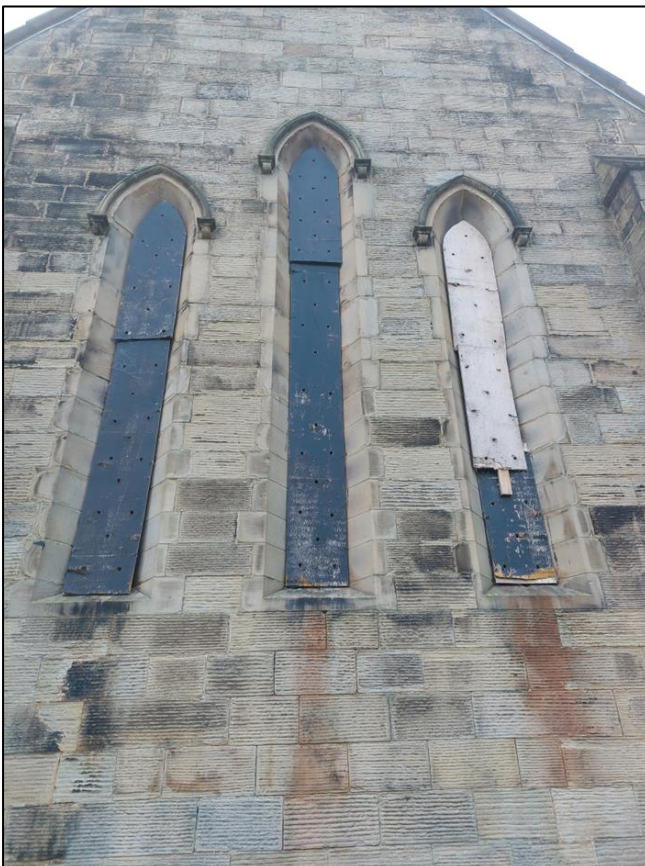
Fig.18 – Corrosion run off from metal shutters to be removed.
