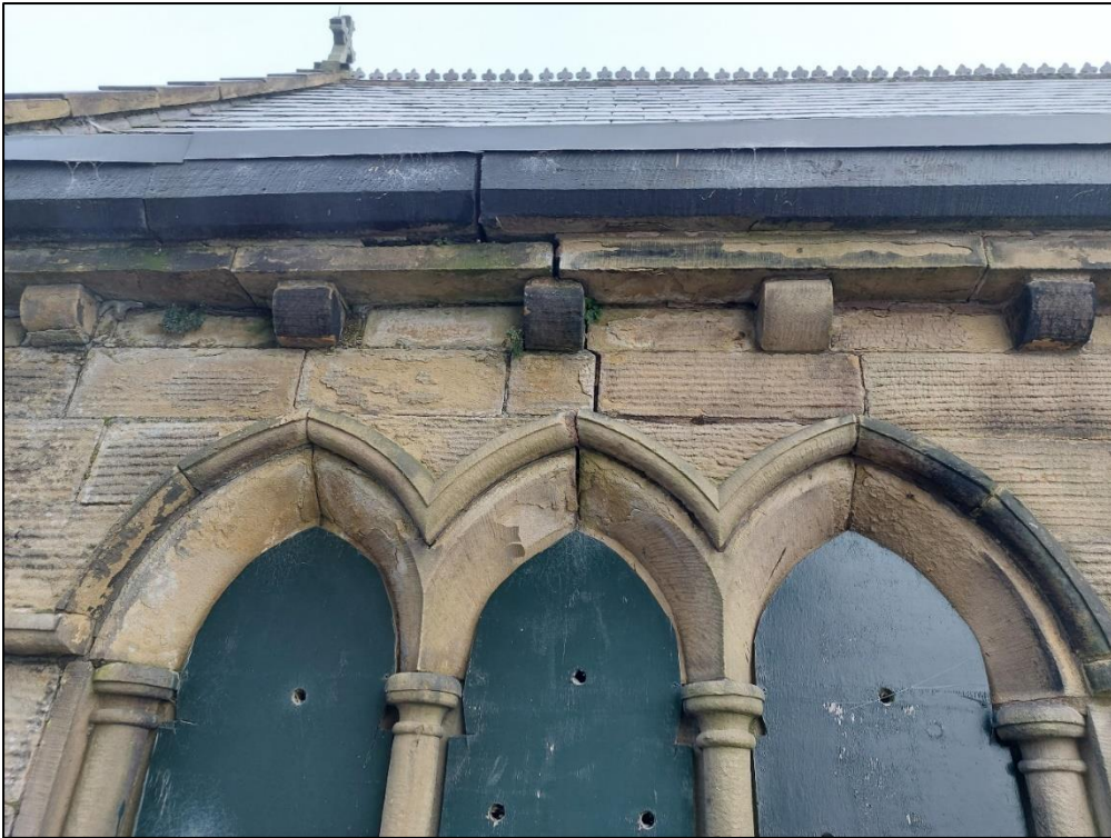
Fig.15 – Open joint above first floor window to south Nave
