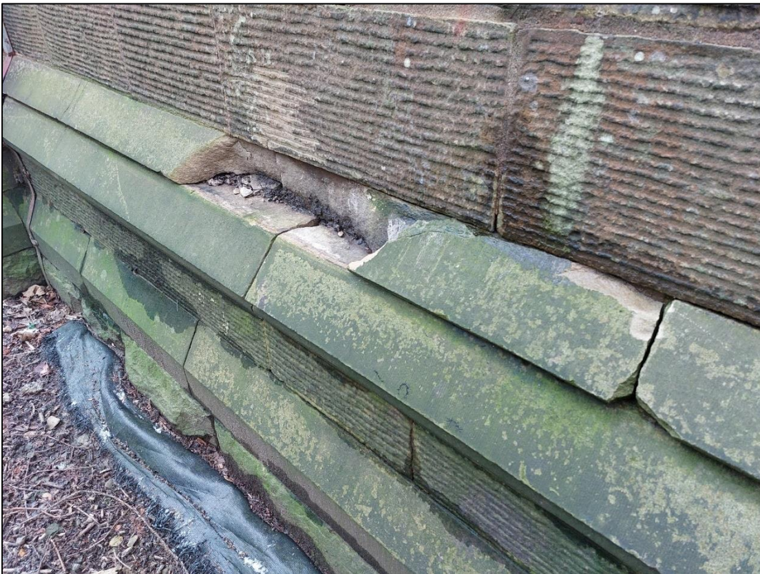
Fig.28 – Missing plinth capping stone to west elevation to tower.
