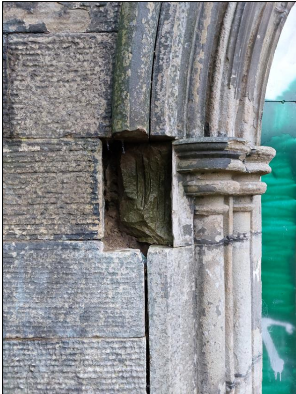
Fig.1 - Missing carving to left hand side to tower door.
