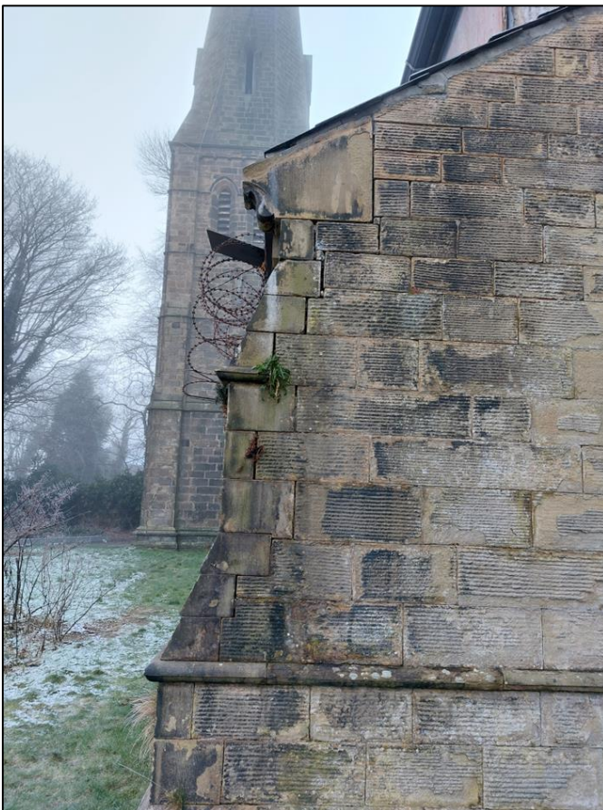
Fig.16 – Open joints between quoins and main wall. Deep pointing to wide joints to quoins. Helical ties if quoins are loose.
