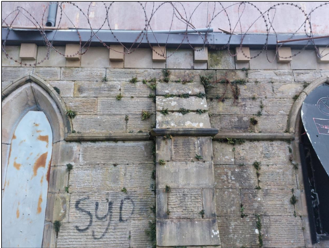
Fig.13 – Algal growth and graffiti to be removed
