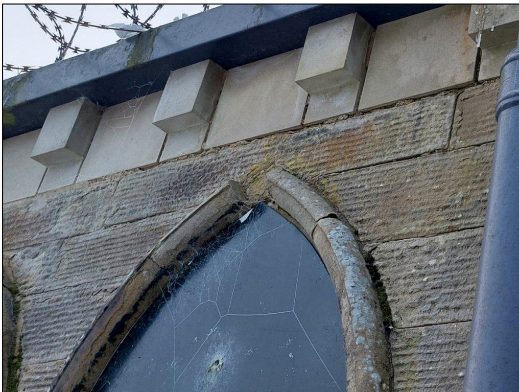
Fig.20 – Missing stone to string detail over windows. New indent repair proposed to reinstate string detail at head of window
