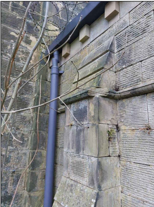
Fig.10 – Lost weather detail to buttress. Indent repair to string detail around buttress
