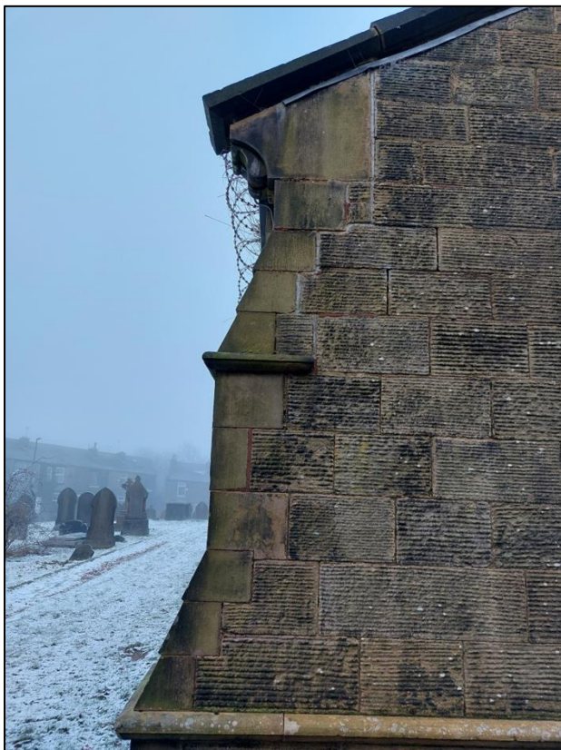
Fig.24 – Inappropriate sealant filler to west elevation of north aisle. Proposed to remove and point.
