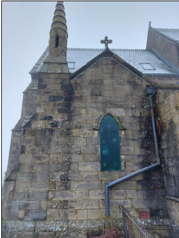
Fig.19 – Soiling following saturation of stone adjacent to guttering. To be manually cleaned/brushed off with water.
