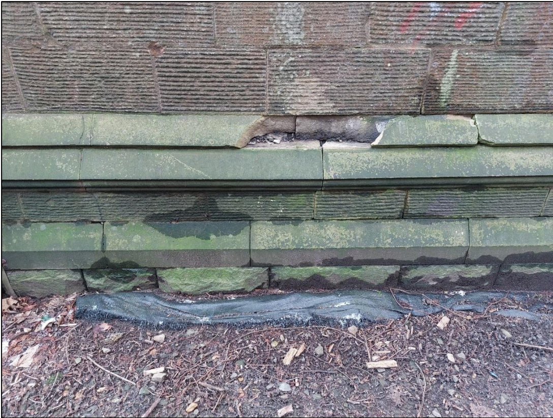
Fig.27 – Missing plinth capping stone to west elevation to tower.
