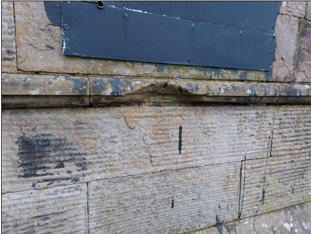
Fig.11 – Loss of section to drip detail. Proposed indent repair to reinstate drip detail.
