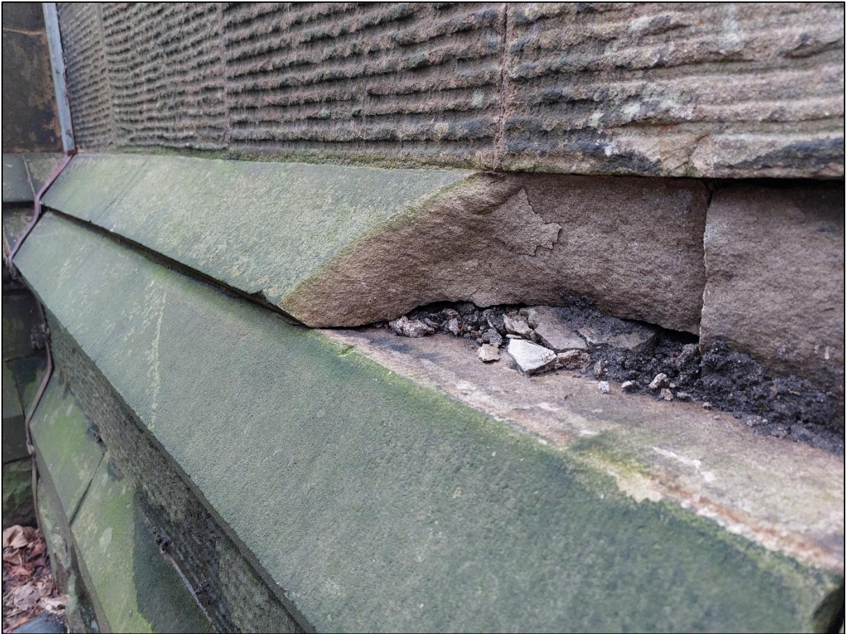
Fig.29 – Missing plinth capping stone to west elevation to tower.
