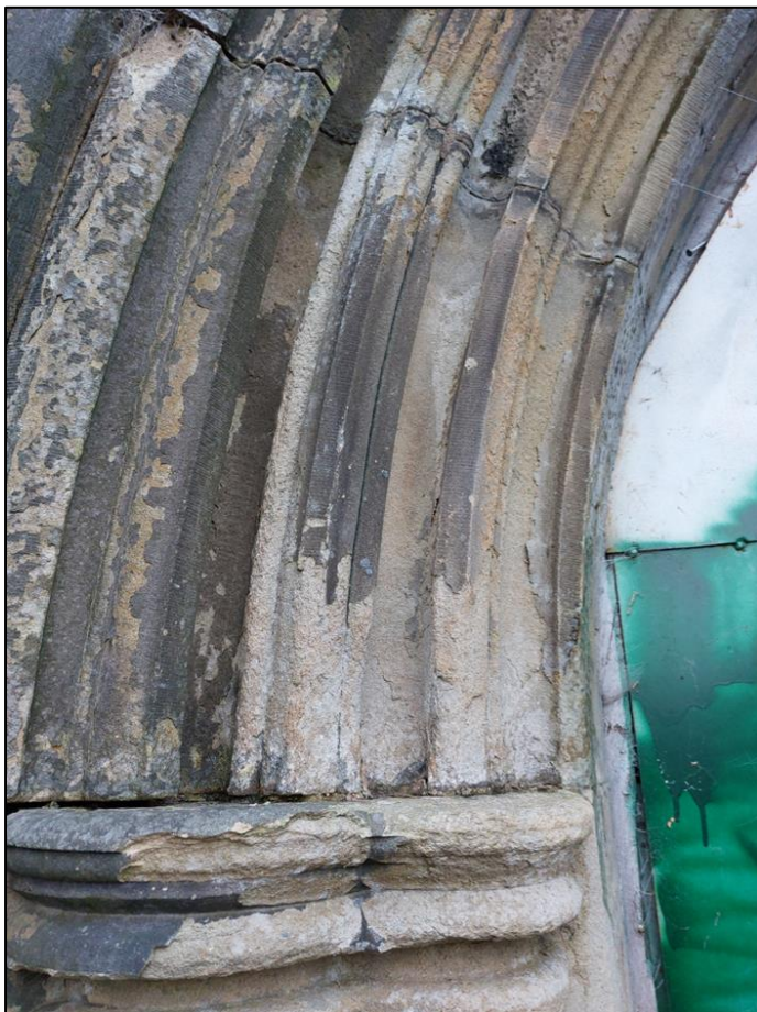
Fig.6 – General weathering and loss of section to stonework to Tower arch, contour scaling, missing pointing. De-frass and pointing of joints proposed.
