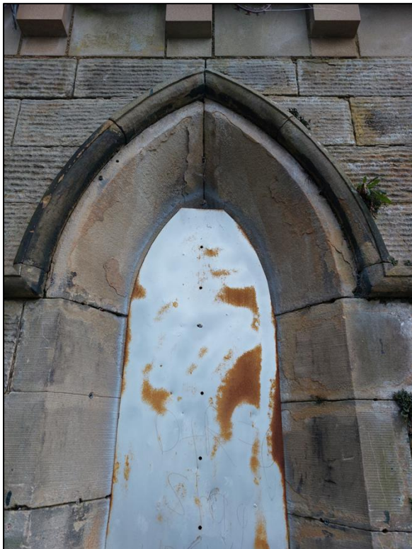
Fig.14. Contour scaling to chancel door. De-frass.
