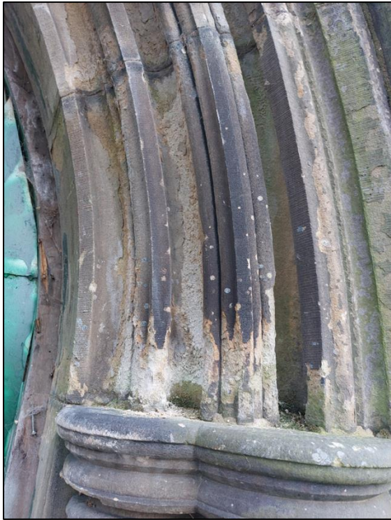
Fig.5 – General weathering and loss of section to stonework to Tower arch. De-frass
