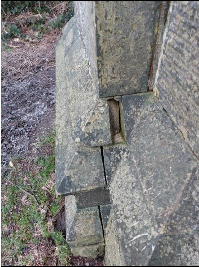
Fig.3 – Indent repair required adjacent to tower door opening.
