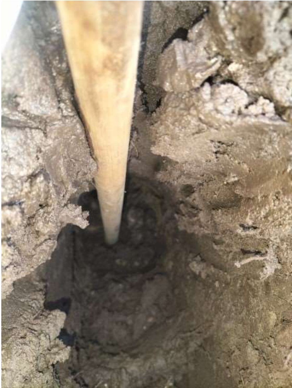
Hand dug pit HDP1, Plot 6.
