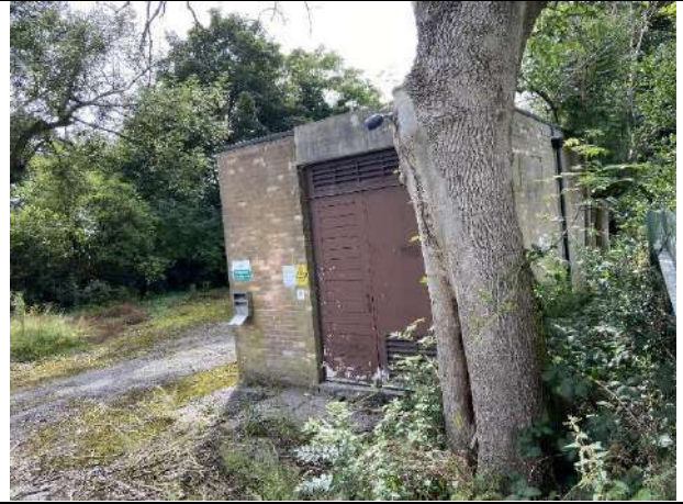
P2: Sub Station in north-west of the site.
