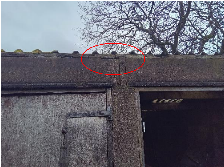
Figure 28. Crevice between concrete and metal sheet roofing.
