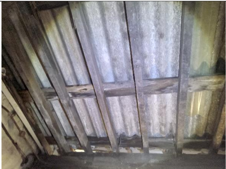
Figure 19. Asbestos sheet roofing.
