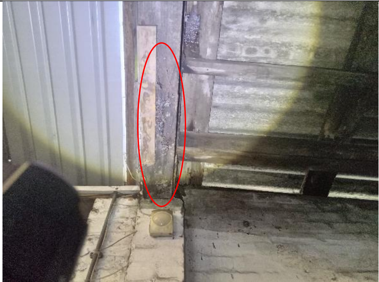
Figure 17. Crevice in wooden beam.
