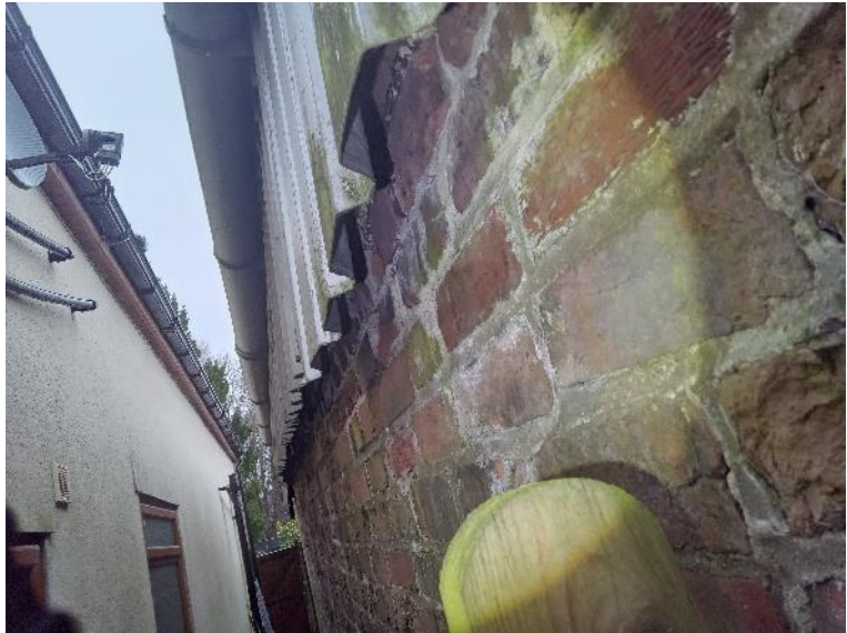
Figure 14. Gap between metal cladding and brickwork.
