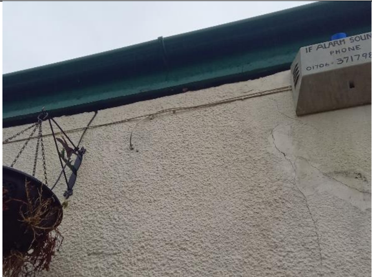
Figure 11. Gap between supporting wall and fascia.
