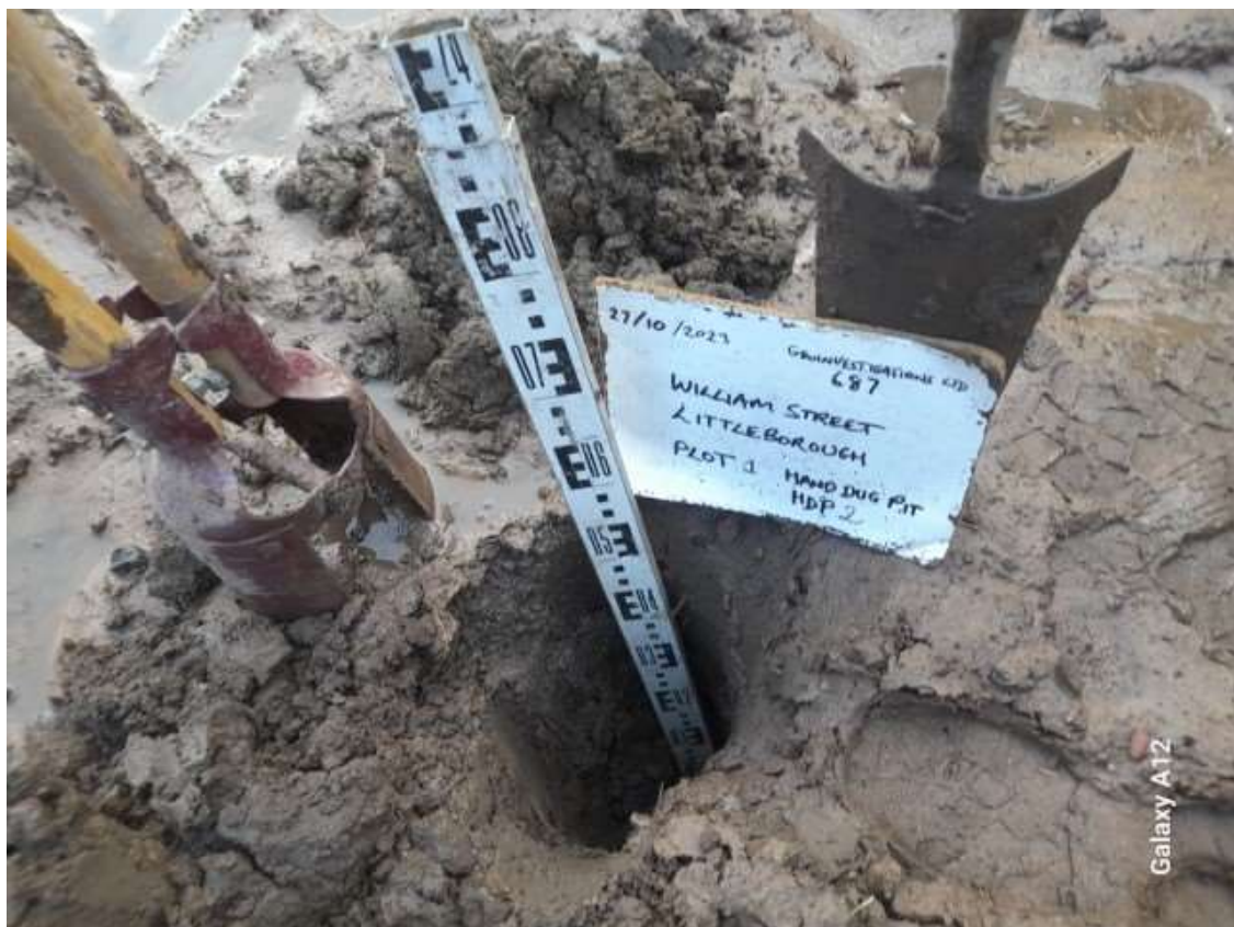
Hand dug pit HDP2 (Plot 1).
