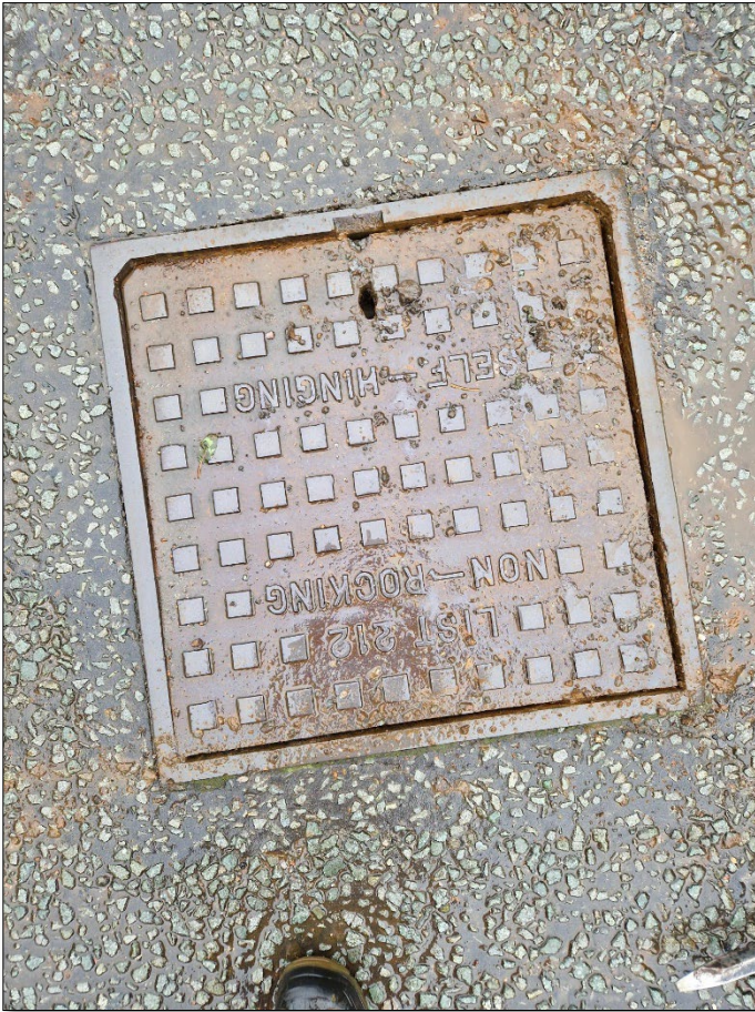
MH2 Cover Condition View
