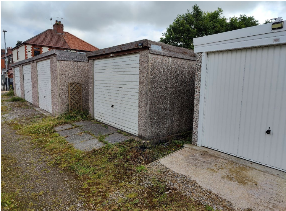
Photograph 4: Garages in the east of the Site (in relatively good condition), facing northeast.
