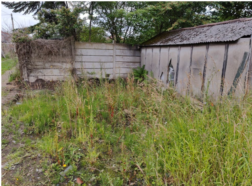
Photograph 12: Overgrown vegetation and garage in relatively poor condition in the north of the Site, looking north.
