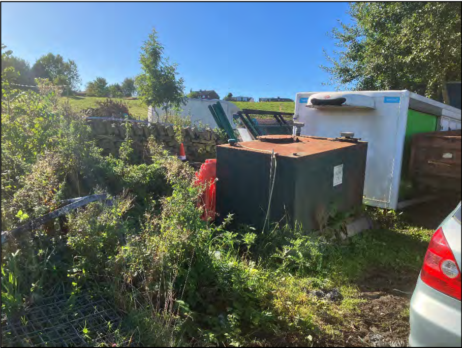
Photograph 2: Oil tank at Cleggswood Farm.
