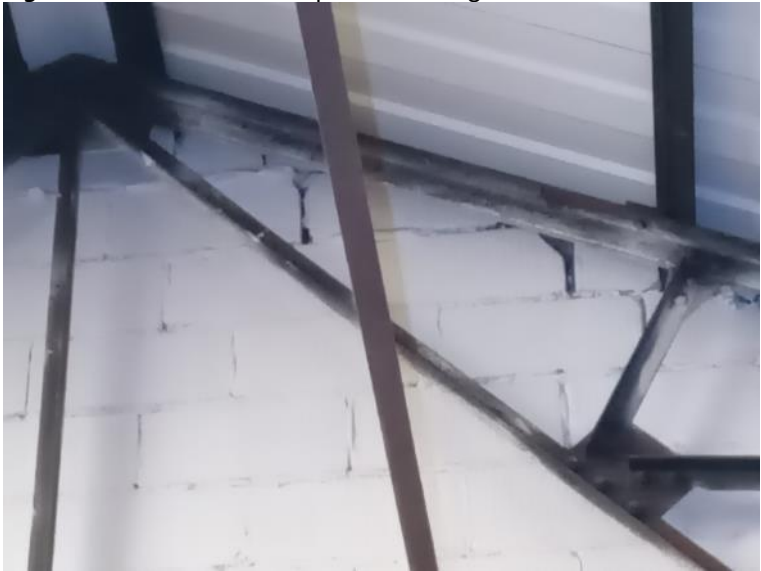
Figure 23. Slight crevices between mortar and brickwork – internal western gable.
