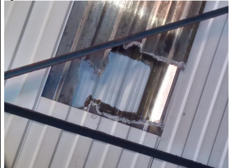
Figure 17. Hole in skylight.
