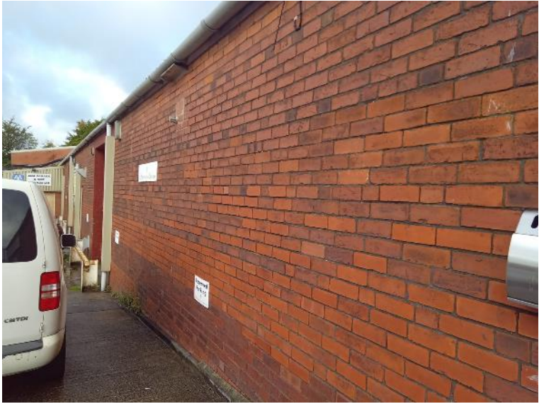
Figure 7. Rest of supporting wall intact.
