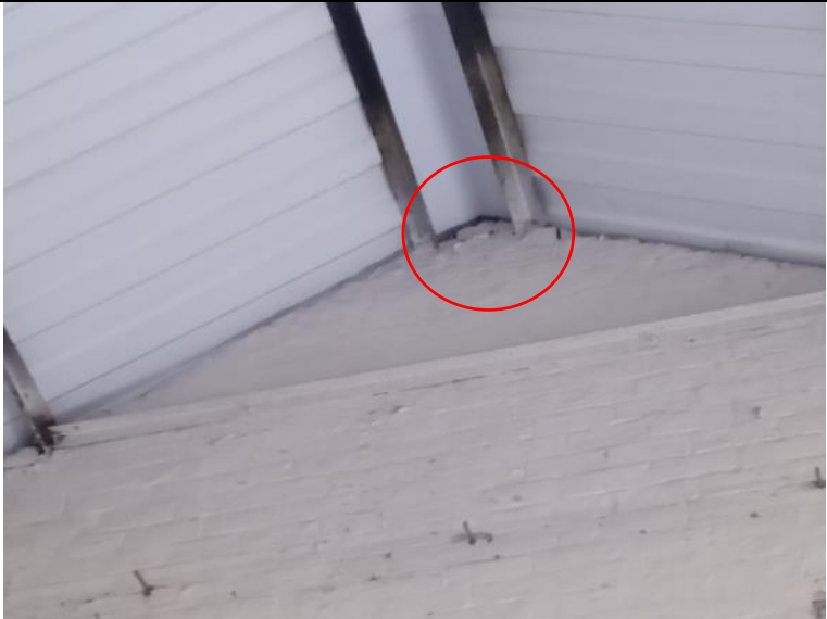
Figure 24. Crevice near apex – internal eastern gable.
