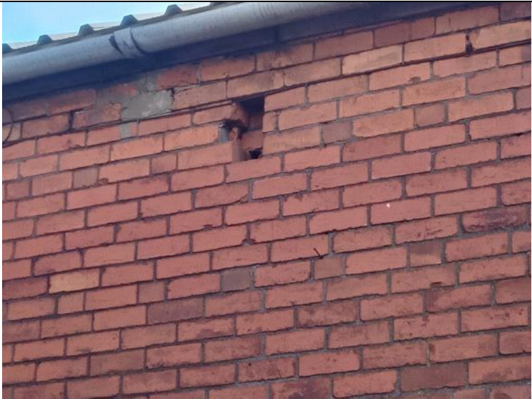
Figure 6. Missing brickwork in supporting wall.
