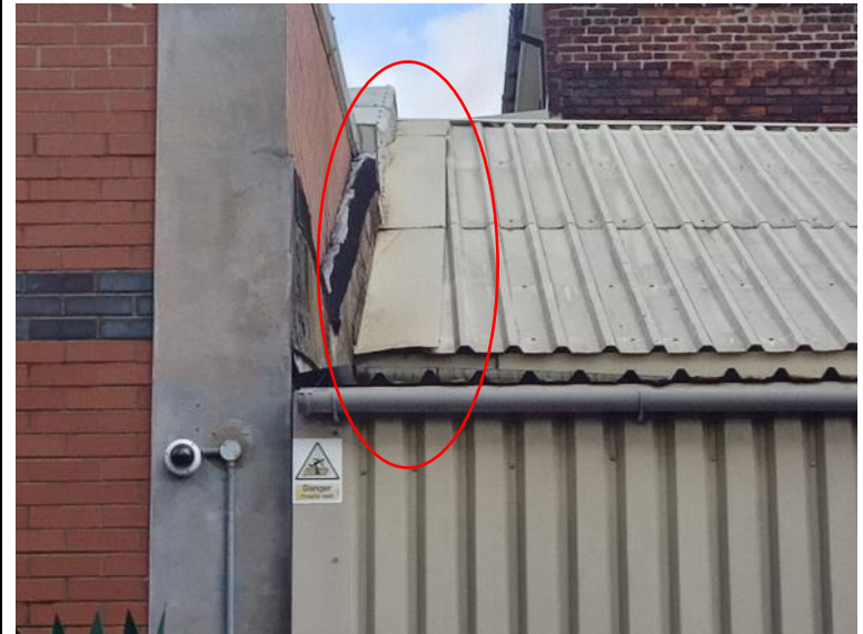
Figure 5. Gaps on southwestern corner.
