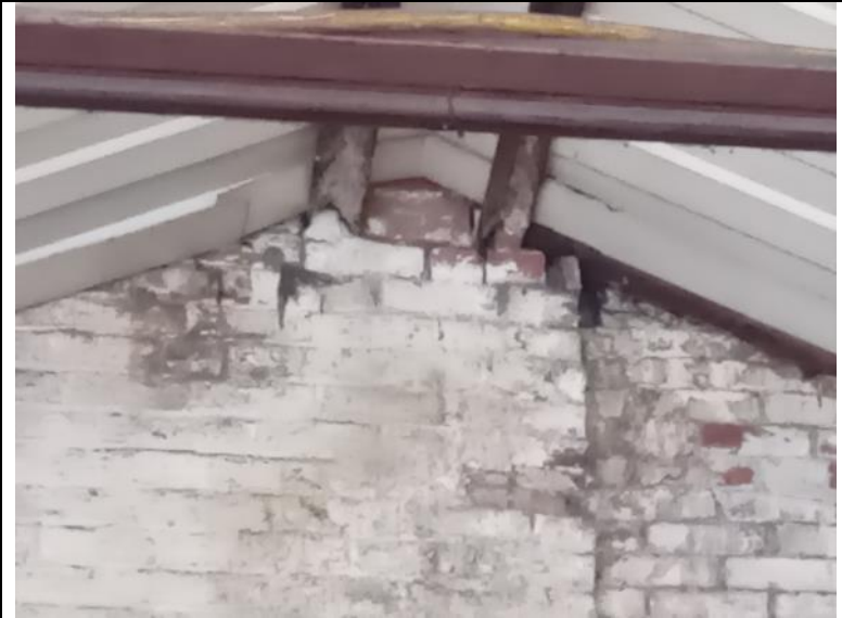
Figure 16. Crevices between mortar and brickwork – internal western gable.
