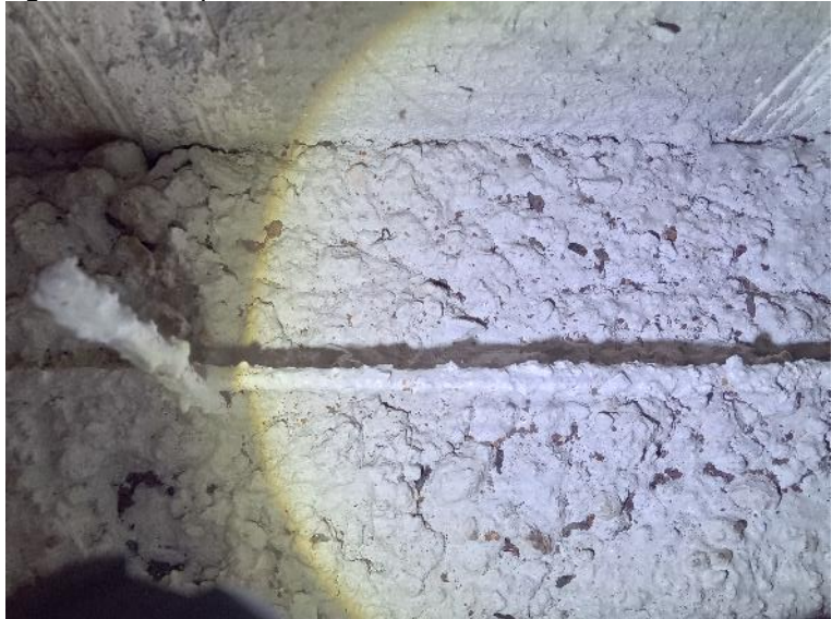
Figure 27. Mouse droppings in cement-filled cavity wall.
