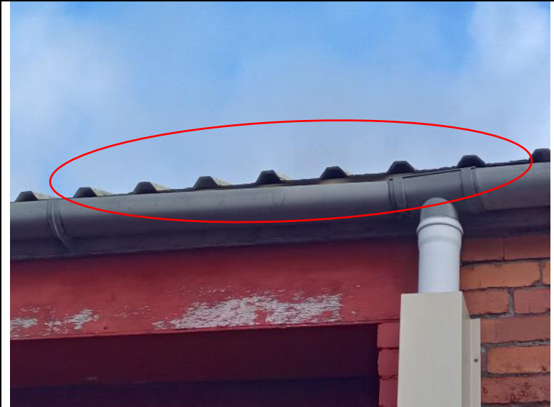
Figure 4. Gaps in roof sheeting at eaves.
