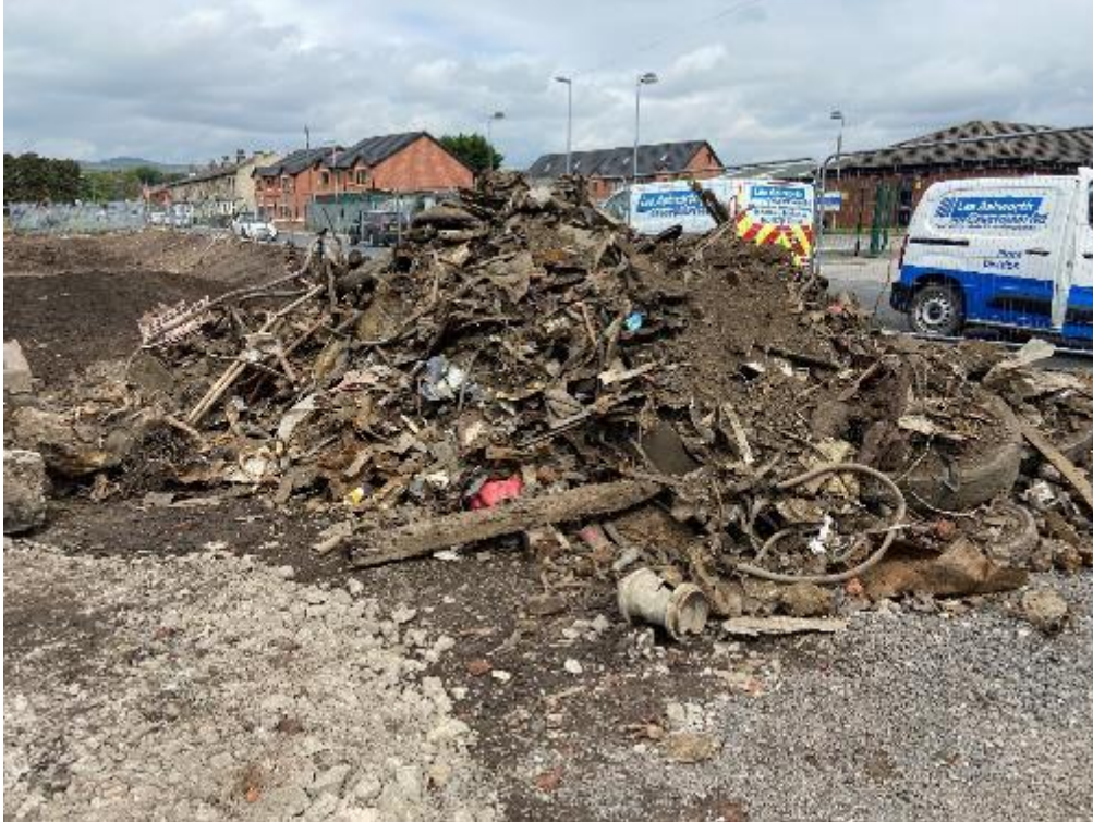
PLATE 11 STOCKPILE OF FRAGMENTISER WASTE IN SOUTHEAST CORNER OF SITE PENDING OFF-SITE DISPOSAL (FACING NORTH)
