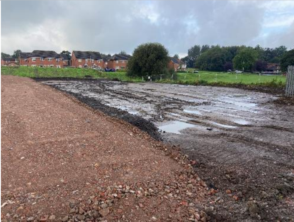
PLATE 22 SOFT SPOT LOCATION FOLLOWING BACKFILL AND COMPACTION (FACING NORTHWEST)
