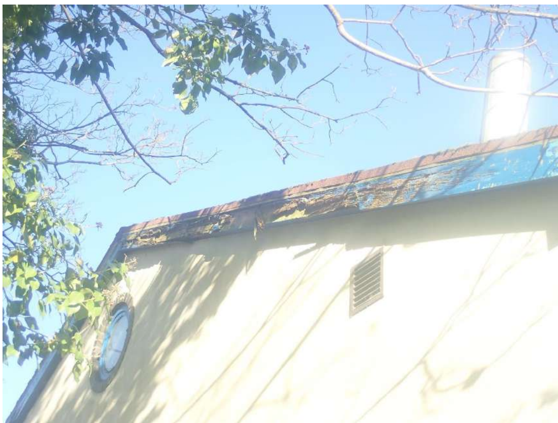
Photograph 5 – Damaged soffit on the single-storey gable.
