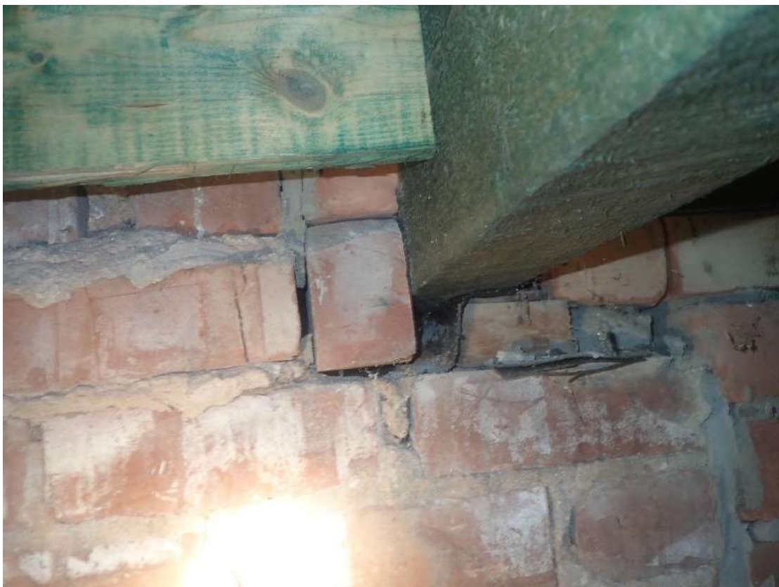
Photograph 14 – Crevices in brickwork in the crawl space under the building.
