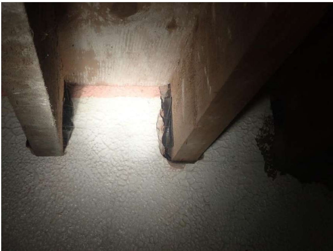
Photograph 12 – Gap around timber beam on the building's ground floor.
