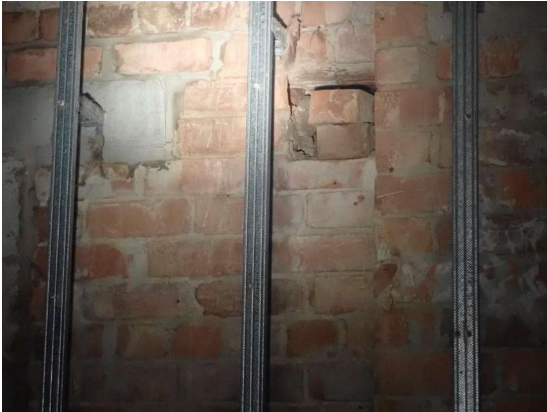
Photograph 11 – Gap in the brickwork on the building's first floor.
