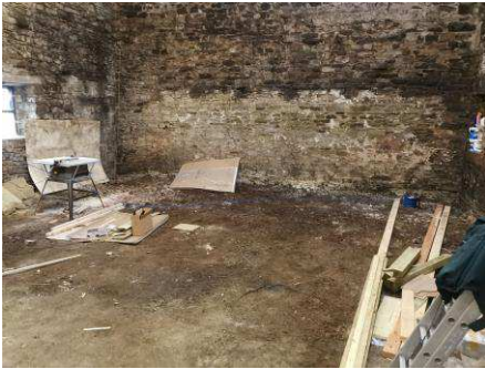
Photo 1. Exposed soil ground to barn interior.
