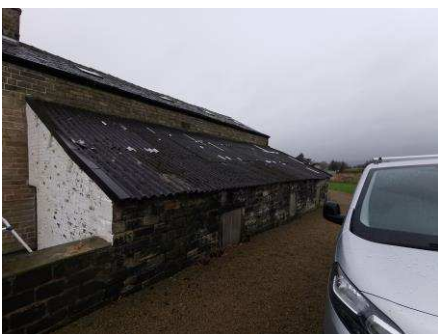
Photo 10. Rear NE elevation showing asbestos board roof to outrigger.
