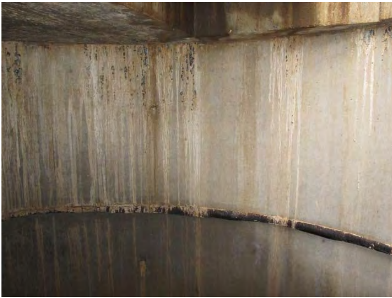
View from Level 1 of MH rings showing infiltration.
