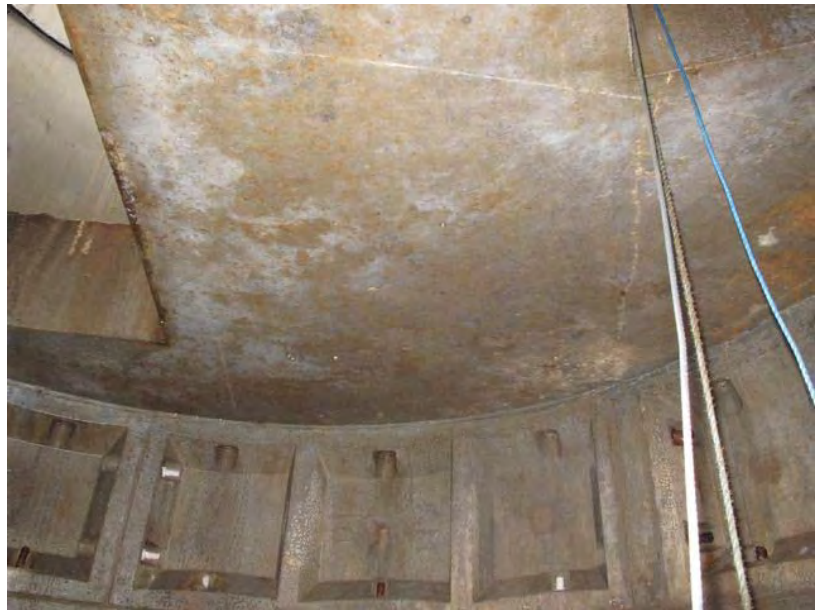
Views from Level 2 Landing Showing Debris, Ladders and Cover Slab above.
