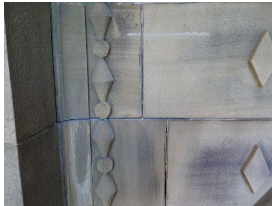
Joints cut out to the decorative facing stonework
