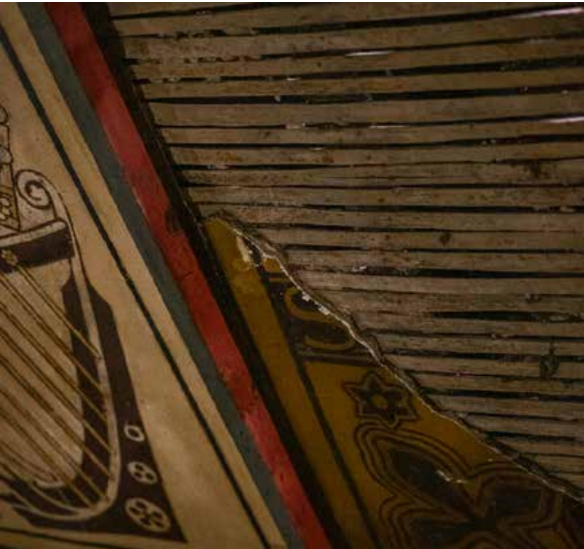
3.1 Damage to one of the Plaster Panels to the Great Hall
