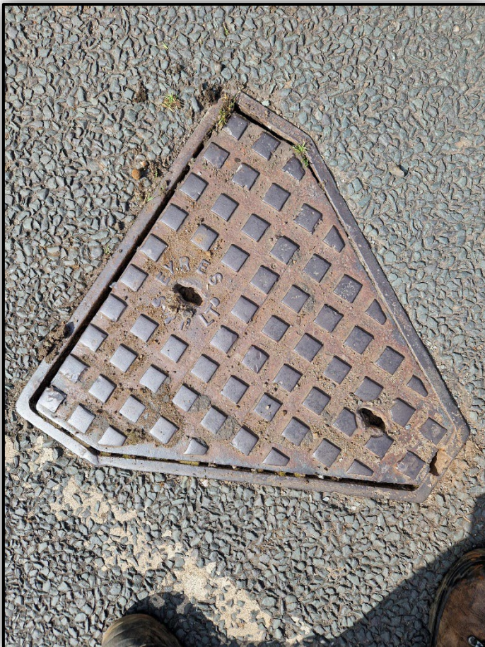
S2 Seized Manhole Cover
