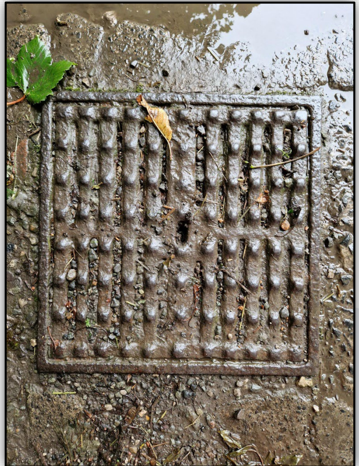
C5 Seized Grated Manhole Cover
