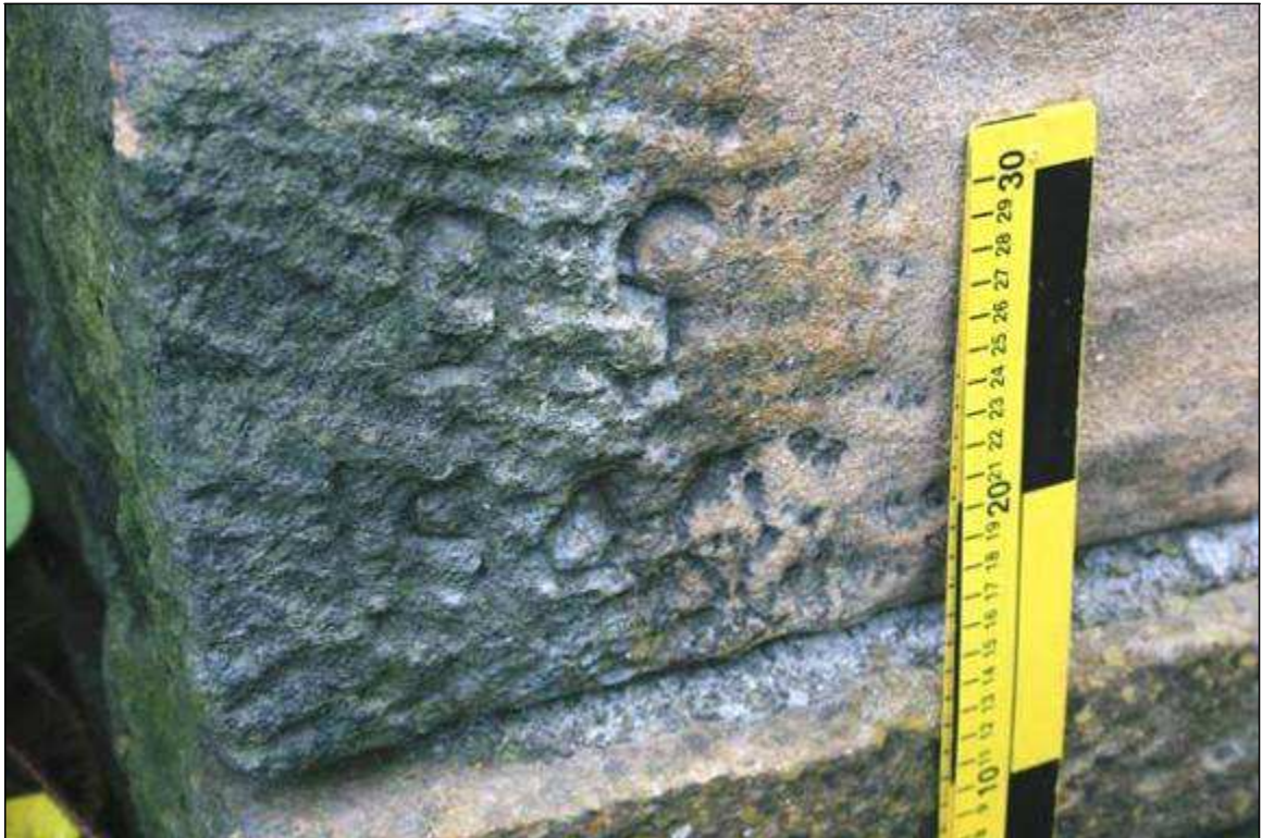
19. Quoin at northwest corner of basement with graffiti initials BS and date of 1900 or 1909
