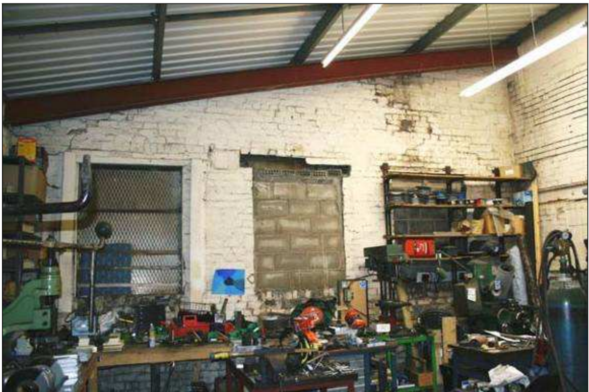
23. Blocked openings in southwest outer wall of outshut
