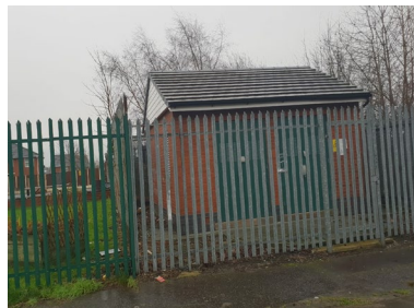
Fig 08: Substation along Joseph Street.
