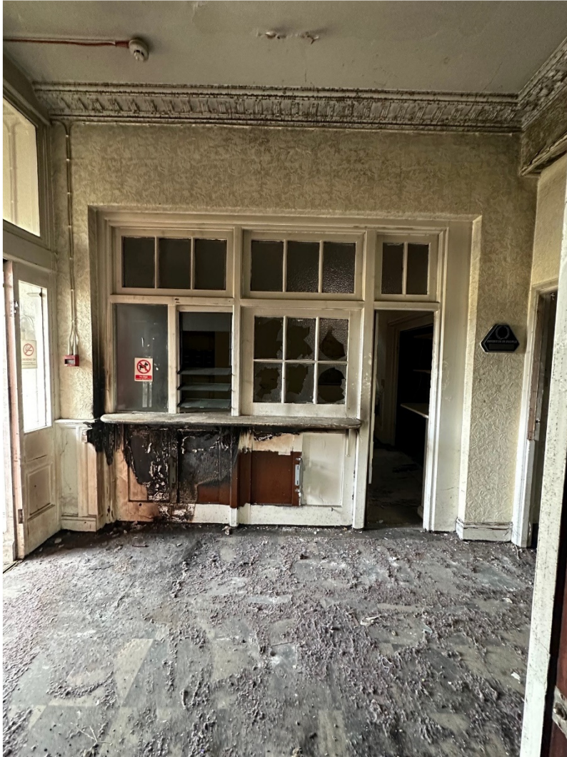
3. Reception screen with admin room
