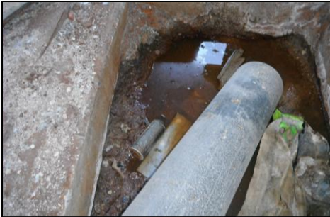
Pit with minor slick to surface in original mill building (Building 7).
