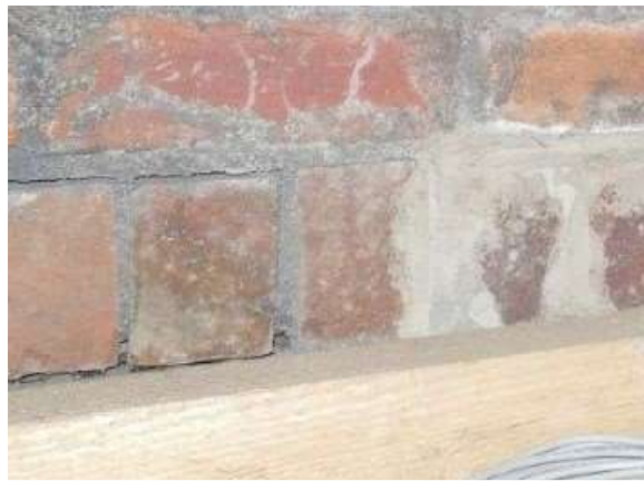
Within the roof void behind the compromised gable there is visible cracking at the base of the compromised panel that appears to coincide with the plane of the fracture externally.
