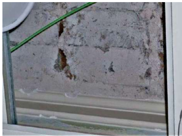
Spalled facing and corroded filler joists. The original coving remains above a recent suspended ceiling. Repair is recommended.
