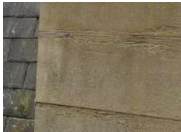
Deterioration of the stonework adjacent to the cement pointing shows where water has remained trapped in the stonework and has frozen. These require very careful raking out.
