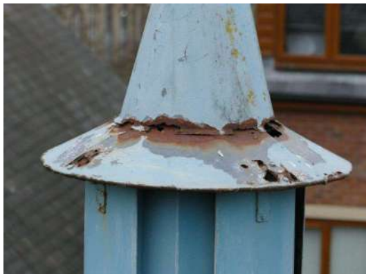
Steel turret cap heavily corroded. Appears to be mild steel replacement of original but not wholly clear. Removal required for repair and re-coating
