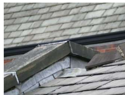
Flashings have a minimal lap and are vulnerable to heavy rain..
