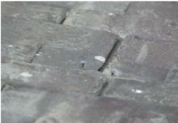
Missing slate from the east slope exposing the joint and nail fixings below. Repair is required..
