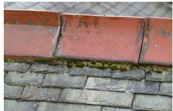
Open joints and split bedding to ridge tiles. Past use of different section ridge tiles for repairs.
