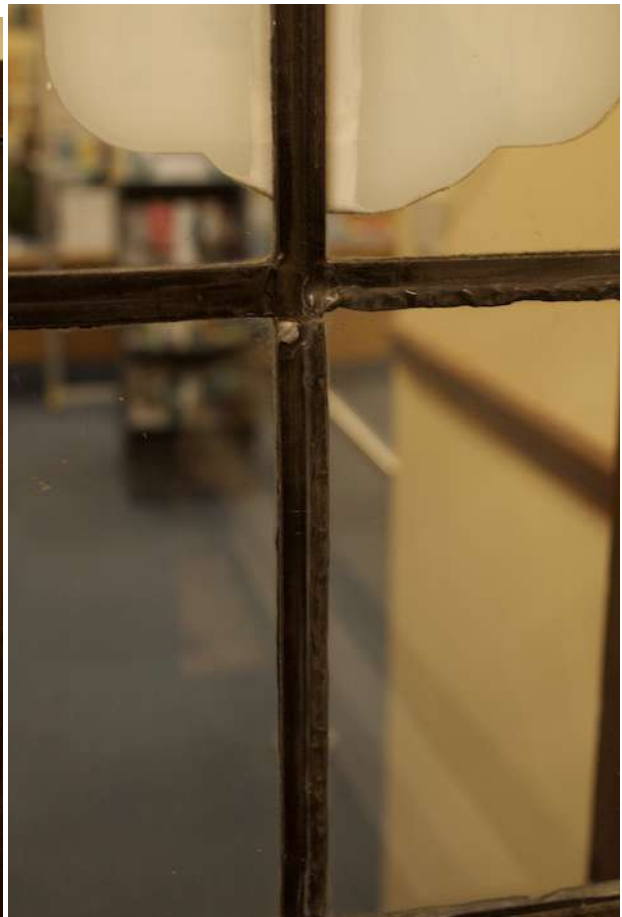
Loose lead in door panel
