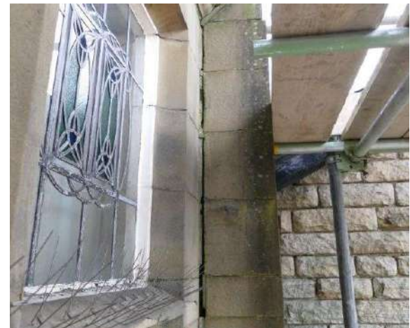
Displaced pier stonework to side of entrance gable. Visible displacement from window head
