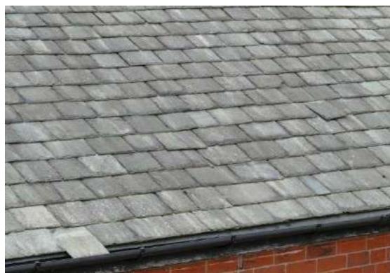
South several slipped slates and several with initial lamination or splits (south slope)
