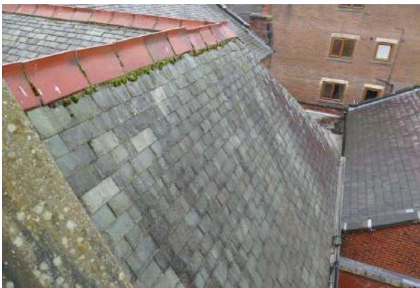
Slipped slate visible in gutter. Spalled/shaled slates and displaced ridge slate. Mis-match in clay ridge tiles.
