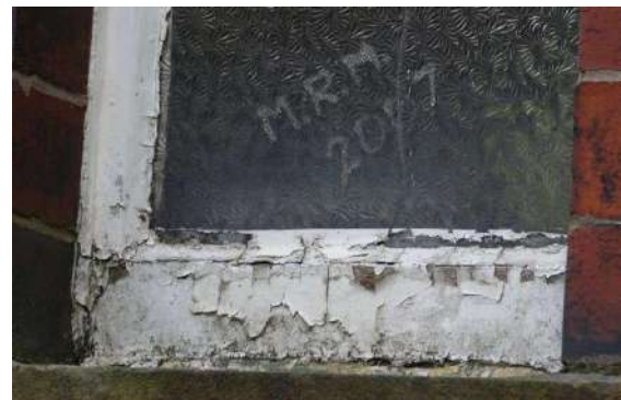
Cill timbers and the lower side of the rails have suffered most from degradation.
