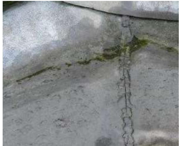
Split in weld to gutter liner from thermal movement of excessively long lead sections with no provision for movement.
