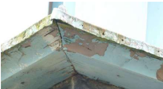
Spalling paint and bare timber to turret base. There is no drip throating in the timber base. Some timber repairs may be required.
