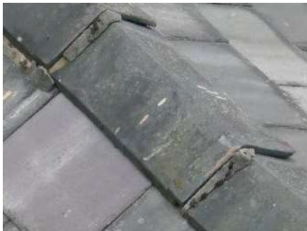
Loss of ridge pointing and bedding mortar.
