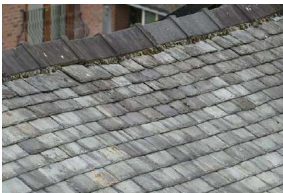
There are two distinct dips in the line of the ridge. It is not wholly clear if these were present during the 2000 refurbishment.
