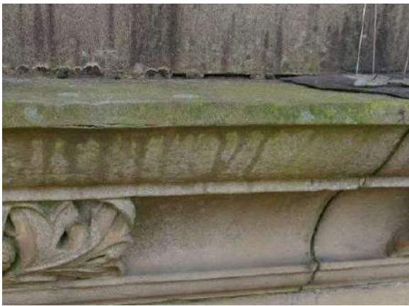
External open joint to the stair window head at the base of the loose section of gable panel,. There are also open joints in stonework below where there is extensive water staining internally.
