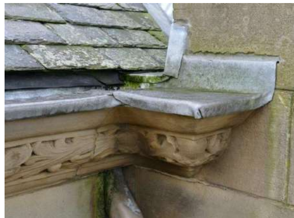
Water ingress around oriel roof gutter outlet. The shallow laps & upstands are likely to be the cause of water leaking through the outlet & staining the stonework.
