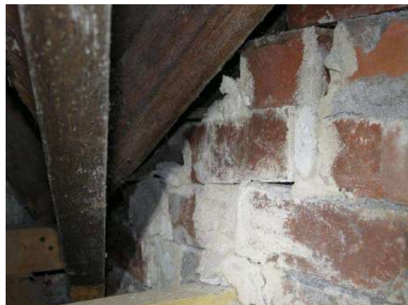
The brickwork to the side of the gable, which coincides with the south east pier and capping, is displaced and lifted. This may have been displaced by the movement in the external pier. This should be assessed during the future dismantling.
