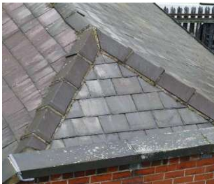
Copings have lead joint flashings but these will hold water as the pointing has in places failed..
