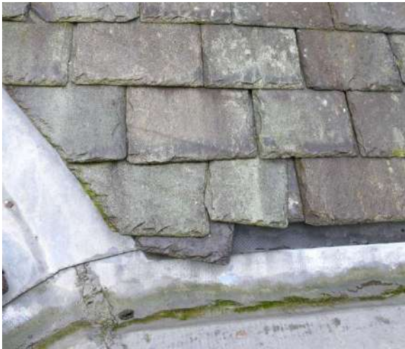
Slipped slates to the foot of the oriel roof/west meeting room roof.
