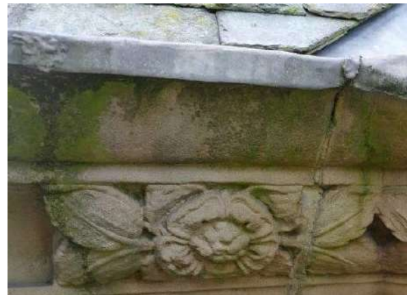
Staining where water has accessed split welds in the lead gutter lining above.
