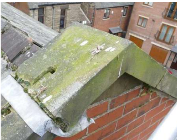
Dog cramps that secured the copings have been removed and the line of the copings appeared to have become a little displaced.
