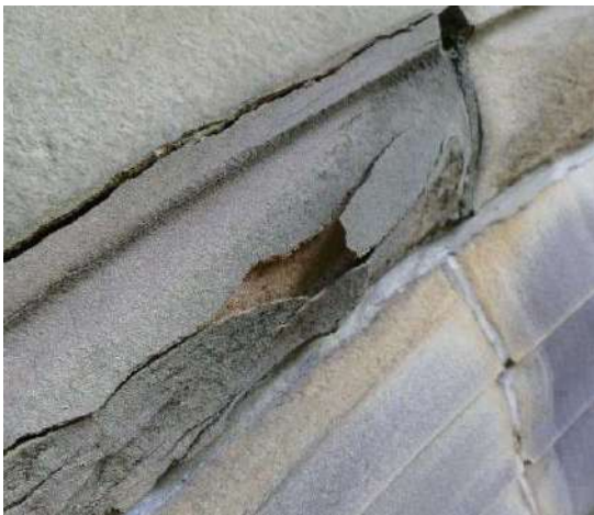
Spalling of stonework adjacent to cement pointing. Raking out strongly recommended.
