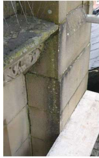
Open joint and displaced masonry to the entrance gable piers..
