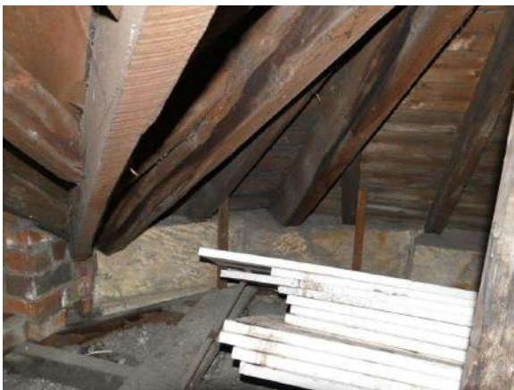
Base of Oriel window north valley. Some water staining to the mitred hip adjacent..
