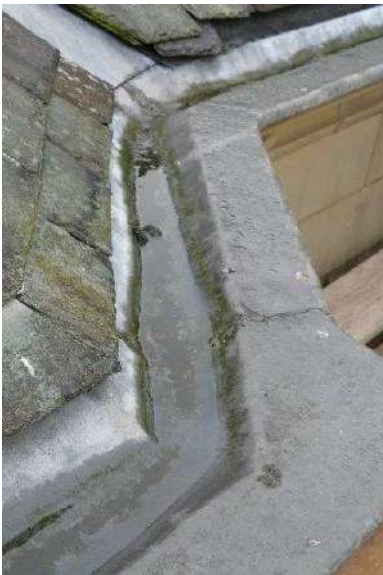
Welded lead gutter lining/apron excessively long and vulnerable to thermal movement. The welded joints show hairline cracks.
