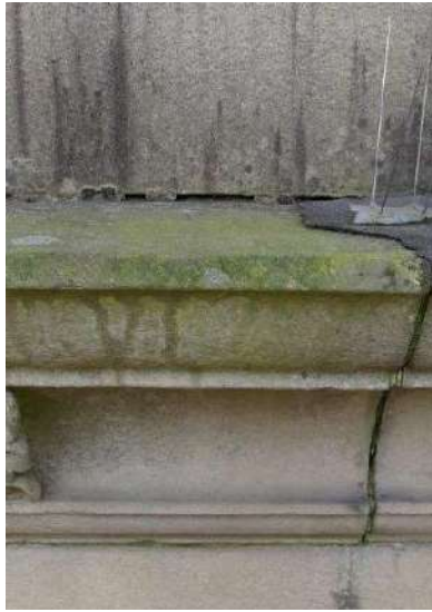
Open joint to the foot of the loose gable panel & window head below.
