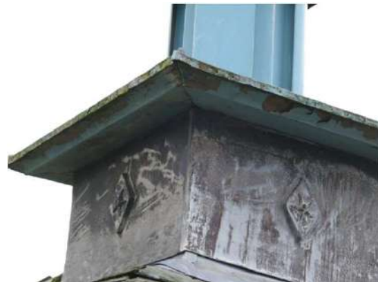
The lead facing to the turret plinth boxing is oxidised and there are hairline cracks and ruffles from thermal movement and tightly dressed corners and fixings.
