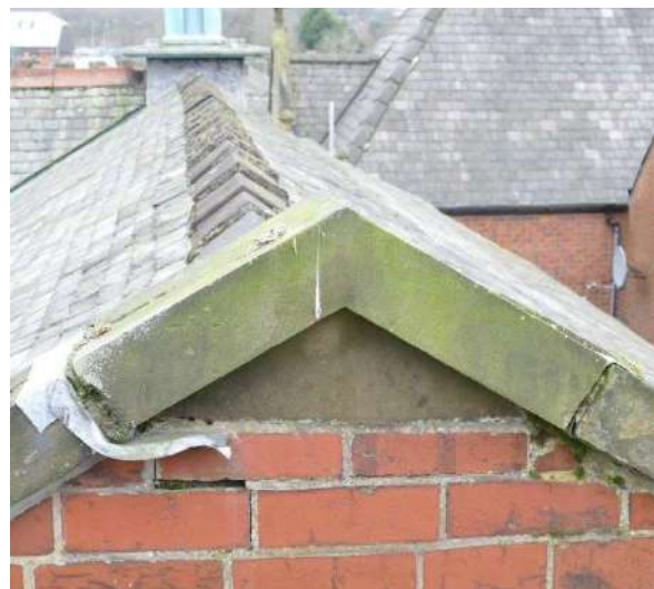
Open joints and partial flashings allow water to penetrate below the copings and damage the mortar.
