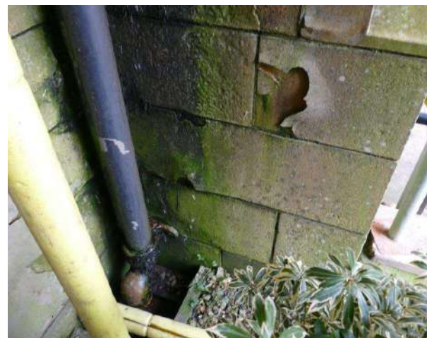
Impact of long term saturation. Rainwater pipe, gully and vegetation all require to be addressed as part of the repair.
