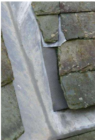
Vulnerable soaker detail and exposed dpc repair vulnerable to UV degeneration.. Possibly also vulnerable to wind blown rain.
