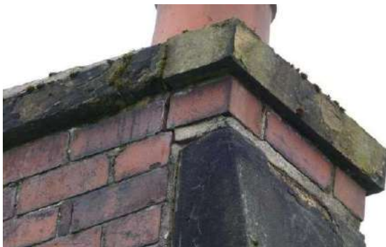
Displaced bricks and capping.
