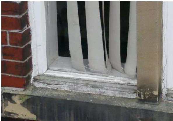
Weathered cill of fixed light window and need for repair and full re-priming and decoration.
