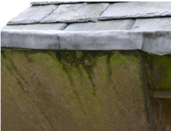
Lead drip capping to oriel window too shallow to fully protect the upper stonework.
