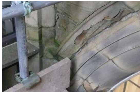
Deterioration of stone facings from saturation below the adjacent flashing detail. This must be addressed to slow the deterioration.
