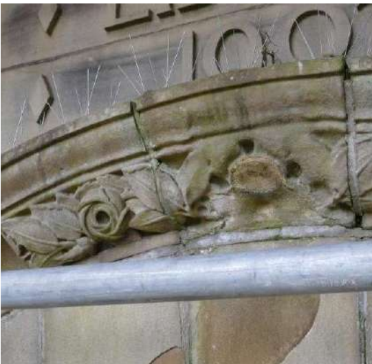
Addressing spalling facings will result in further loss of detail from carved details. New indents to be considered to retain definition.
