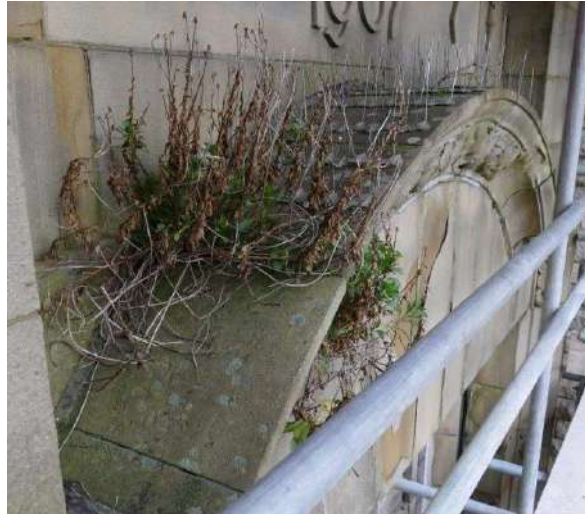
Open joints have been inundated with vegetation which is now causing real damage to the stonework.
