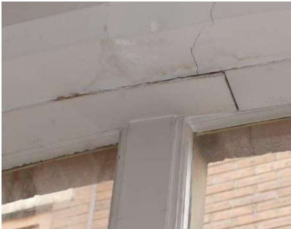
Displaced boarded surround to the east windows and moisture staining of the plaster above. Likely ingress from open joints and copings externally
