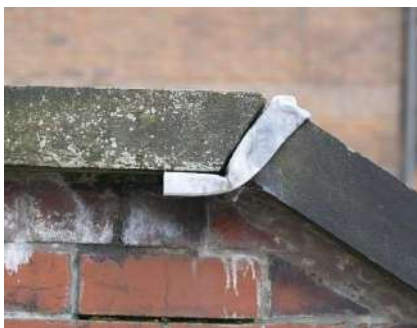
Lead flashing and run off from coping impacting the brickwork.
