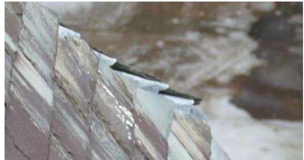
Mitred lead hip detail has lifted leaving the edge slates vulnerable to wind damage. Some re-fixing and re-dressing is now required to ensure integrity.
