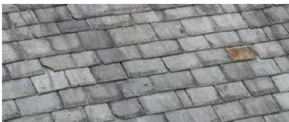
Damaged slates (South slope)
