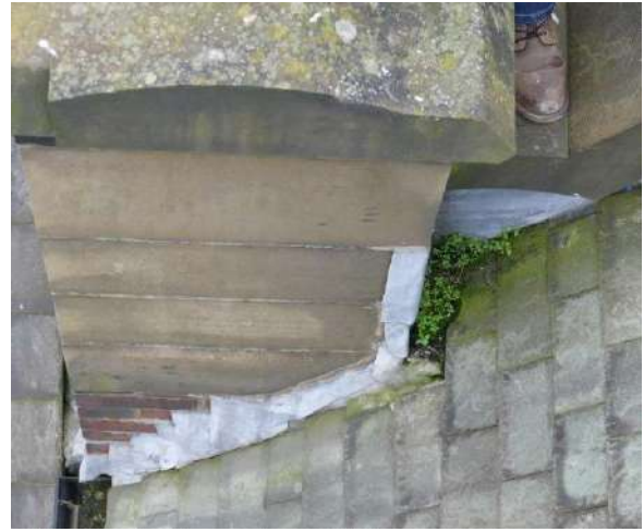
Insufficient lap to soakers/cover flashings where displaced and narrow back gutter blocked with debris..
