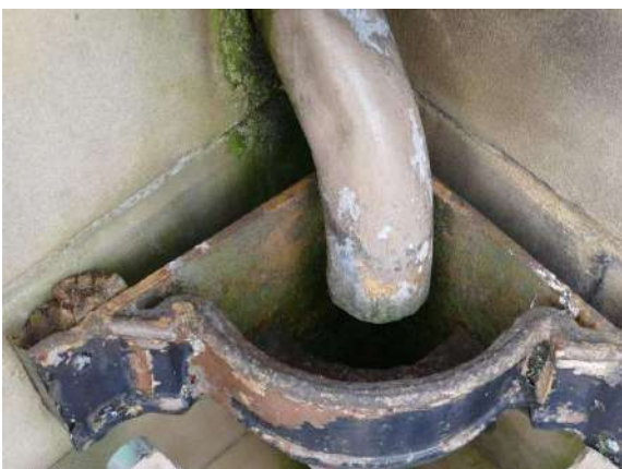
Weathered decoration and rusting of the original cast iron hopper heads. Narrow
