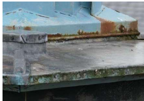
The lower drip detail of the turret is also showing signs of corrosion and fixings may be compromised.
