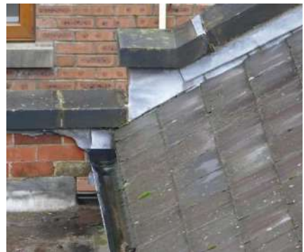
Shallow lap of flashings and vulnerable abutment of wall/coping details
