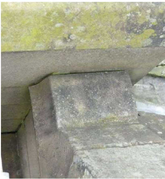
Open joint where the gable panel meets the corner finial. Water can freely run into the joint and into the core of the stone wall.
