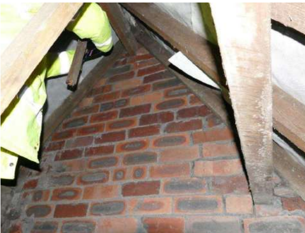
There was no evidence of movement in the internal stretcher bond brickwork. It is possible that ferrous fixings for the stonework have corroded to release the outer panel.
