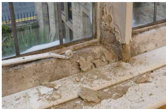
Spalling stone and vinyl paint covering. Consider removing the paint & tidying the stone. Oriel window.
