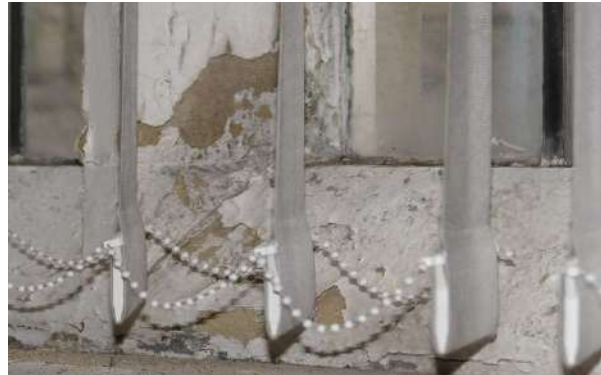
Spalling stone and vinyl paint covering. Consider removing the paint and tidying the stone. Stair window.
