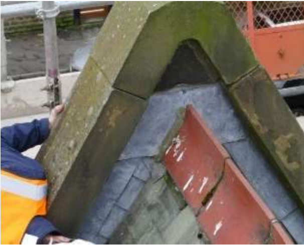
Displaced gable evident in the mis-alignment of the flashings and in the open displaced joint of the coping..
