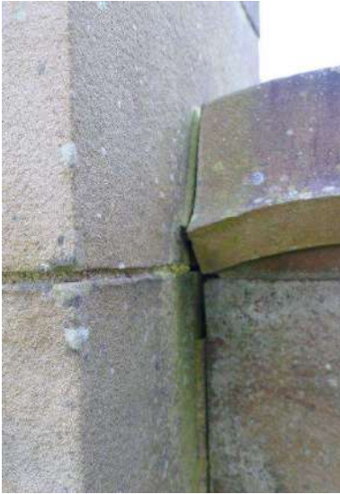
Open vertical joint between copings and buttress finial extended pier.
