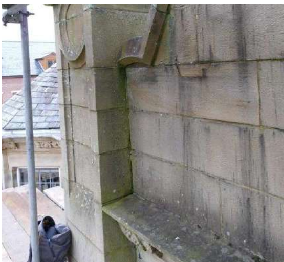
A crack has developed along the junction of the left hand pier and the wall and a significant open joint and displacement to the right hand side.
