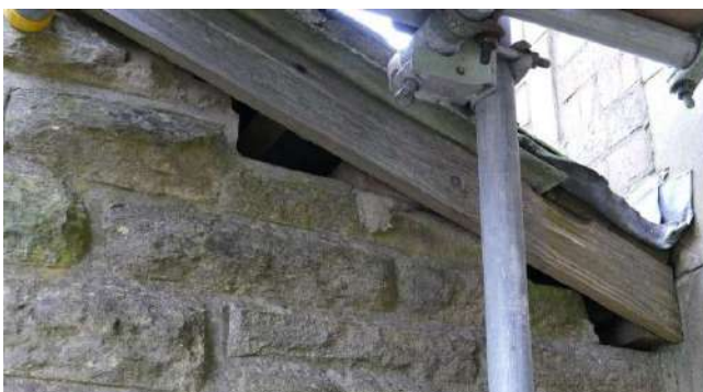
Poorly finished detail to adjoining verge. Open gaps will allow bird and insect access. Poorly finished detail where the back flashing to the abutment meets the verge.
