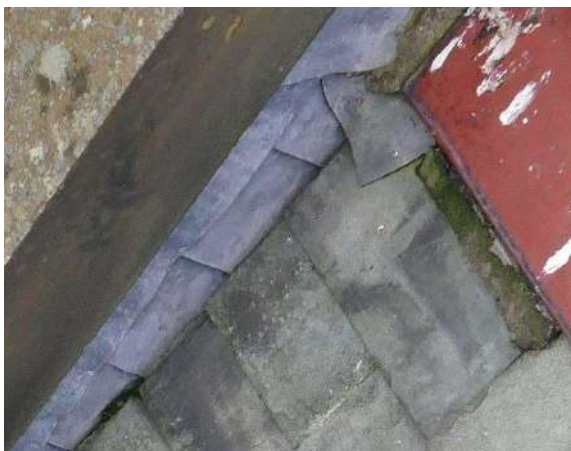
Displacement of the gable appears to have stretched the soakers, reducing their lap with the cover flashings to 30mm in places. This is a likely source of water ingress.
