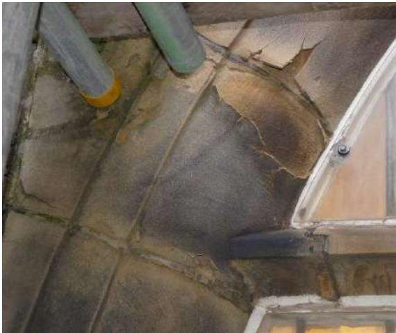
Spalled facing and split to voussoire and past transom repair. Investigation required to assess if full replacement is required.
