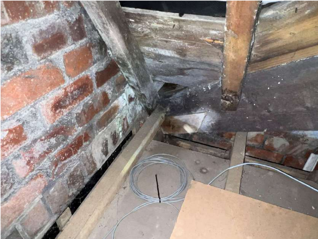
Repaired hip and new ceiling joist above stairs with un-insulated ceiling
