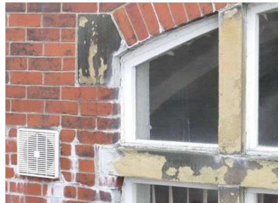
Open joints around casements, extract of warm air that appears to be routed through the chimney flue, cement pointed joints and a lack of drip detailing all appear to have contributed to moisture levels in the wall. The transoms appear to slope back to the frame in places.
