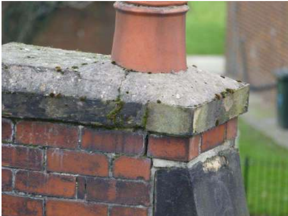
Split in the brickwork, capping and stone facing to the south of the chimney. Open joint from flaunching into the construction.
