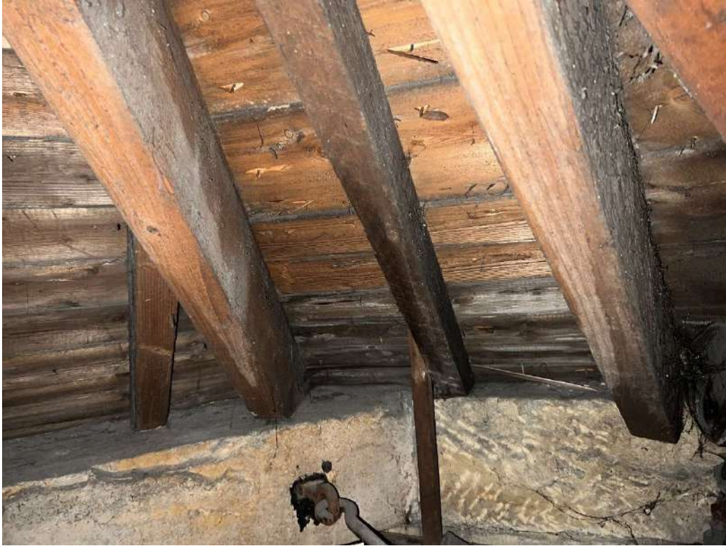
Dry timbers to bay and large member of steel supporting hip to main first floor roof void
