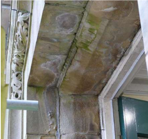
Open joints and displaced spandrel panel above main doorway.
