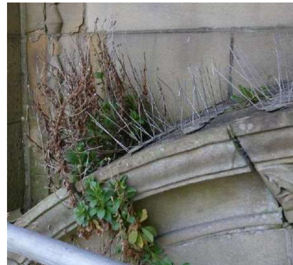
Vegetation and exposed, open joints have led to the local displacement of stonework.
