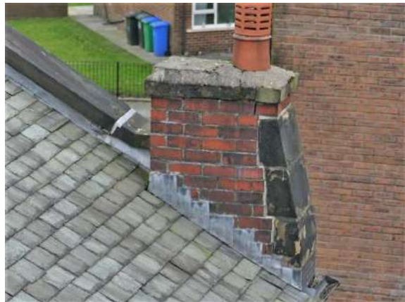
Shallow flashings and outfall detail leaving the chimney vulnerable to water ingress.
