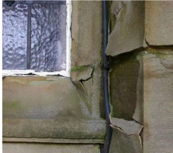
Spalling facings to the pier, stooling, cill and window surround.
