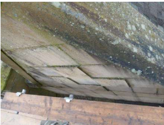
Exposed ledges to the stone detailing relief are vulnerable to standing water and freeze thaw damage. The green algae shows where moisture ledges..
