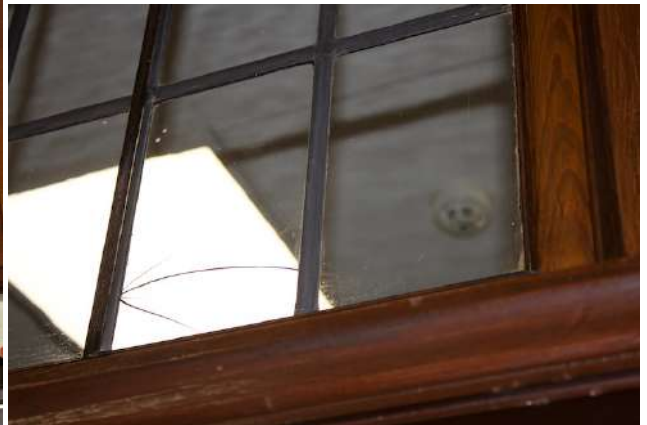
Damaged pane to internal window
