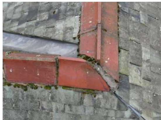
Open joints and split bedding to ridge tiles. Past use of different section ridge tiles for repairs.
