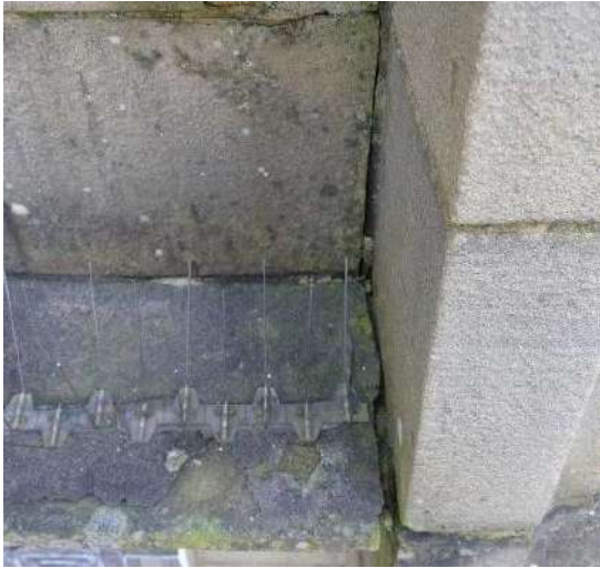
Open joints to the edges of the compromised gable panel.
