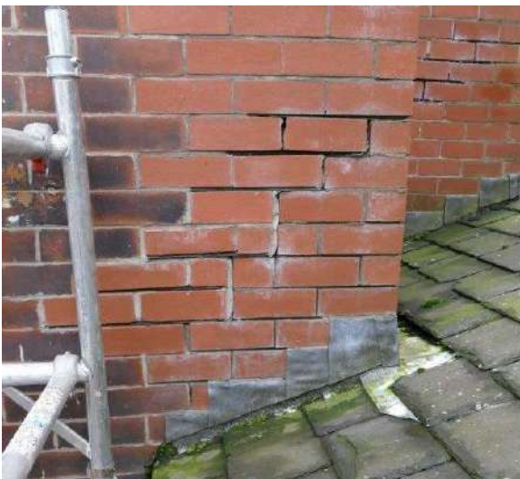
Open joints on stepped cavity tray. Possible settlement of new wall/foundation but requires to be re-packed and pointed.
