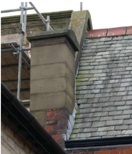
The south pier extension is displaced from the central wall panel and appears to be
