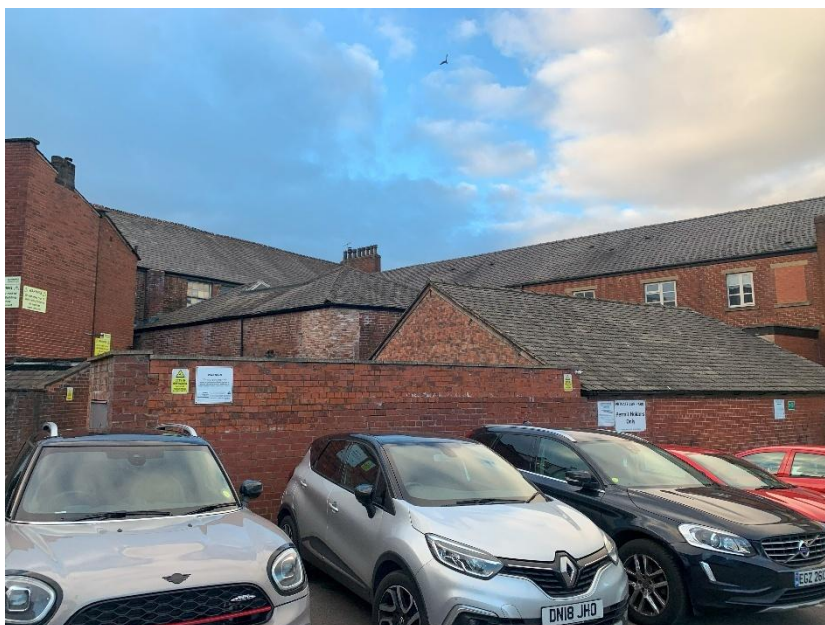
Figure 2.3: Rear elevation showing projecting gables where a roof lantern has likely been removed.
