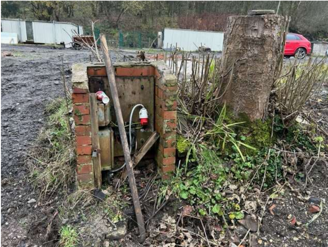
Plate 15 – Housing to three phase electrical supply to former Mill buildings
