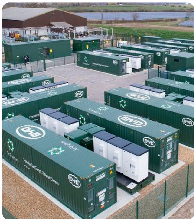
Battery storage units
