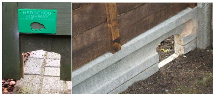
Insert 6: Showing wildlife access gap within fencing
