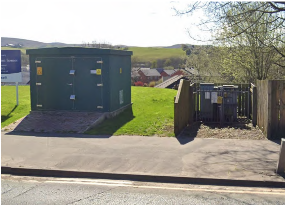
Photograph 6: Google Streetviewer imagery of electricity sub station c. 35m west
