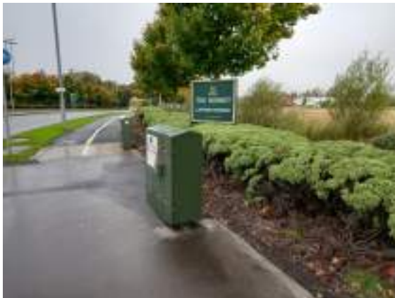
Photo 22— Electricity substation outside of Hornet Pub.
