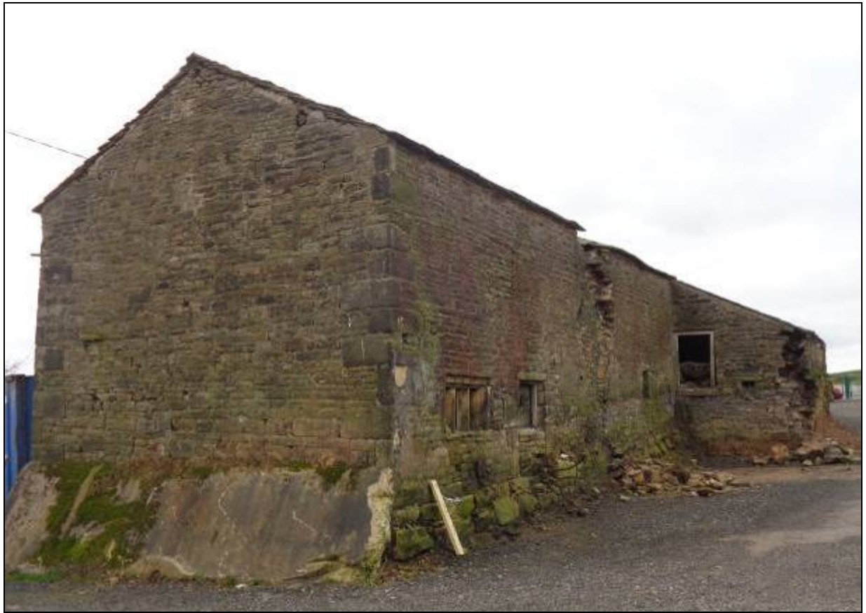
7. Rear elevation has partly collapsed
