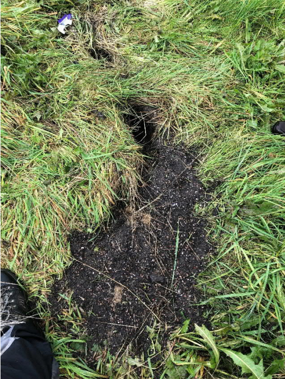
Photo 10: Evidence of infilled ground (2/2)
