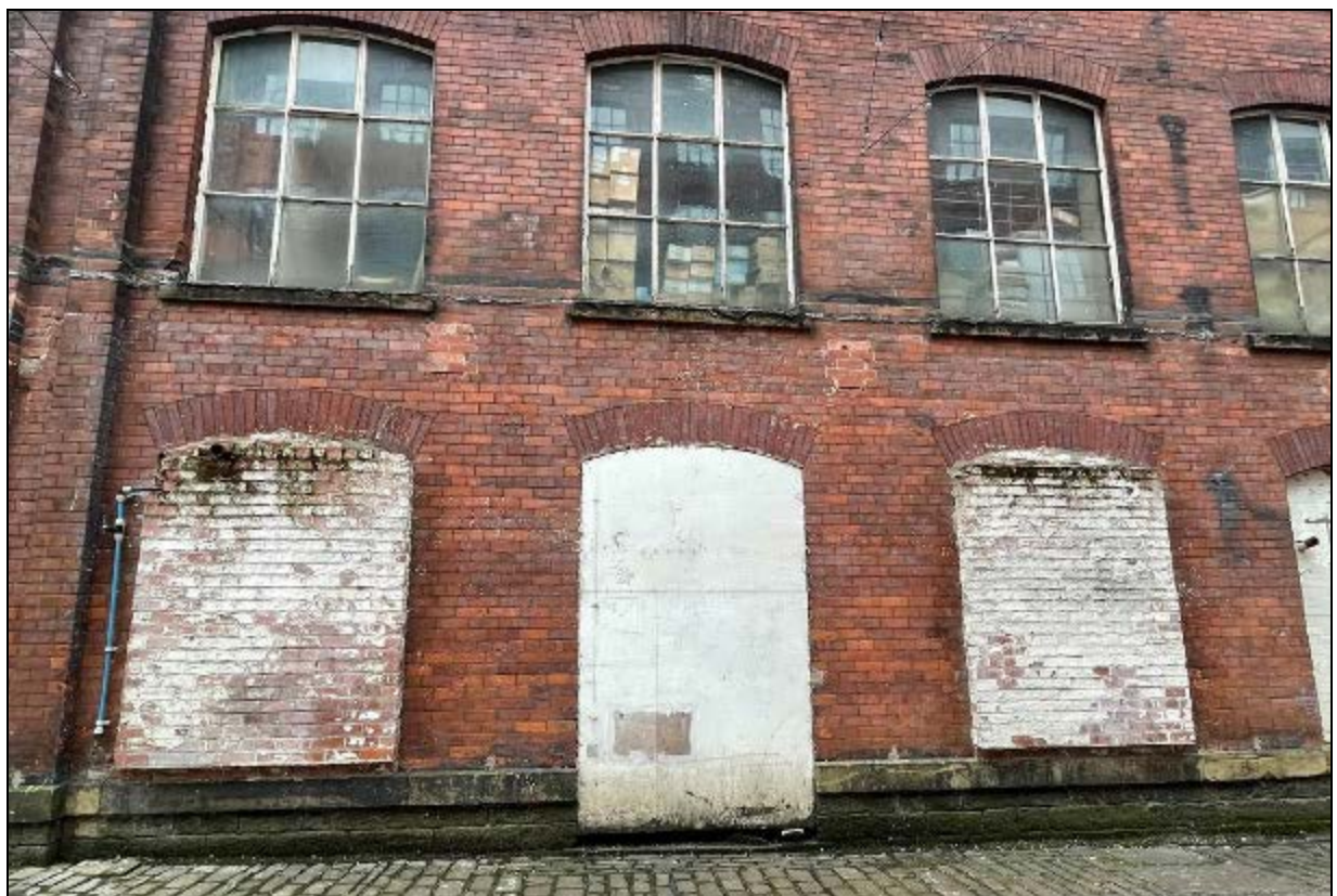
5. Blocked openings in the southwest elevation
