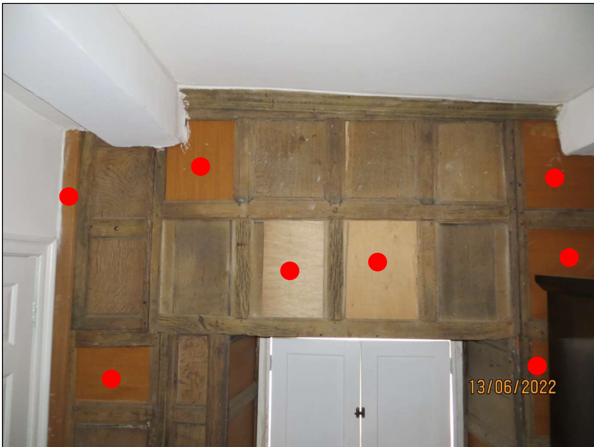
Figure 13: A typical example of a section of the wall panelling. Note the panels that have been inappropriately replaced with plywood (marked with a red dot in this picture).
