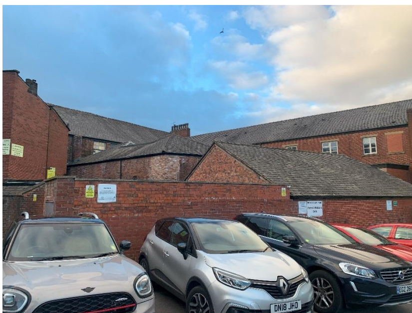
Figure 2.3: Rear elevation showing projecting gables where a roof lantern has likely been removed.
